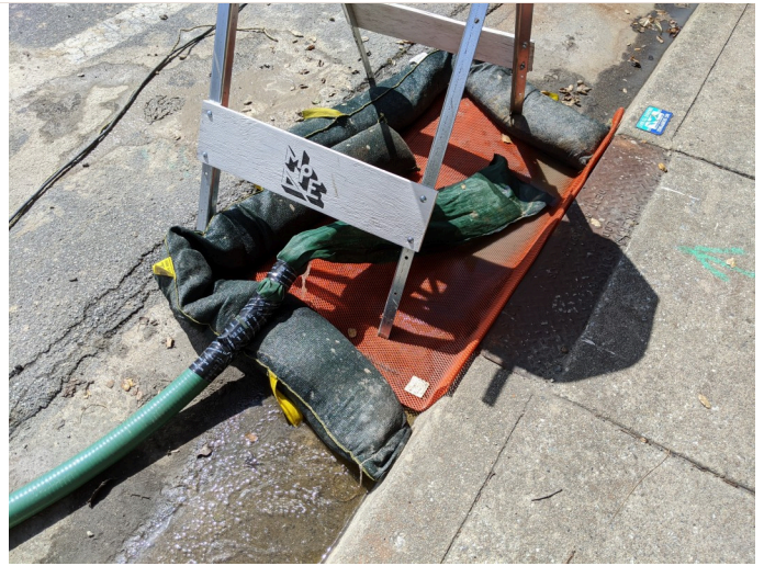
outlet of groundwater sump pump into stormwater drain with silt filter
