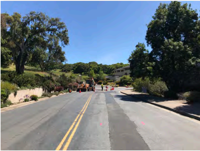
MPE and Cal Am testing the pipeline from an access point located on Blue Larkspur Ln.
