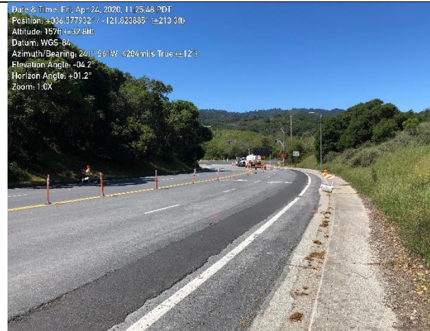
Photo 2. Conditions on Ragsdale Drive.
