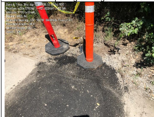
Photo 3. Recently installed Air Release Valve on Ragsdale Drive
