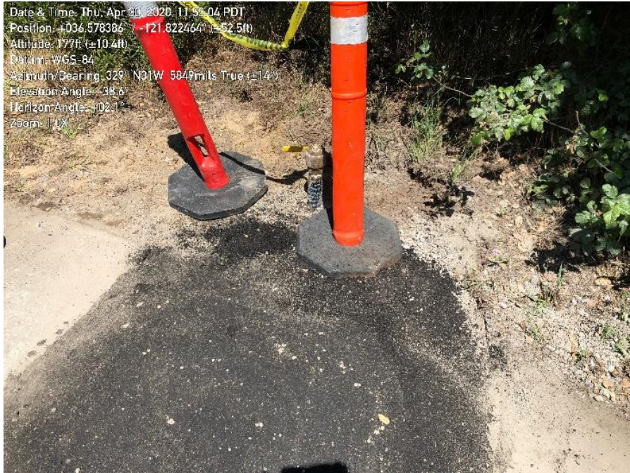
Photo 3. Recently installed Air Release Valve on Ragsdale Drive.
