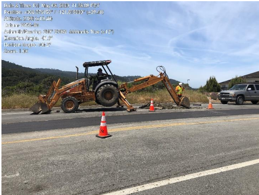
Photo 2. MPE paving repairs on Lower Ragsdale Drive.
