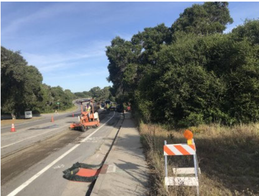
05/06/2020 - Intact stormwater BMPs in use adjacent to construction along Lower Ragsdale Drive during paving activities.
