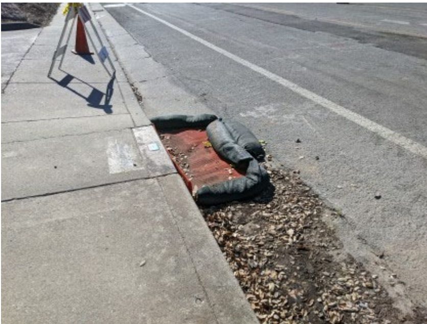
05/04/2020 - Intact stormwater BMPs in use adjacent to construction along Lower Ragsdale Drive.
