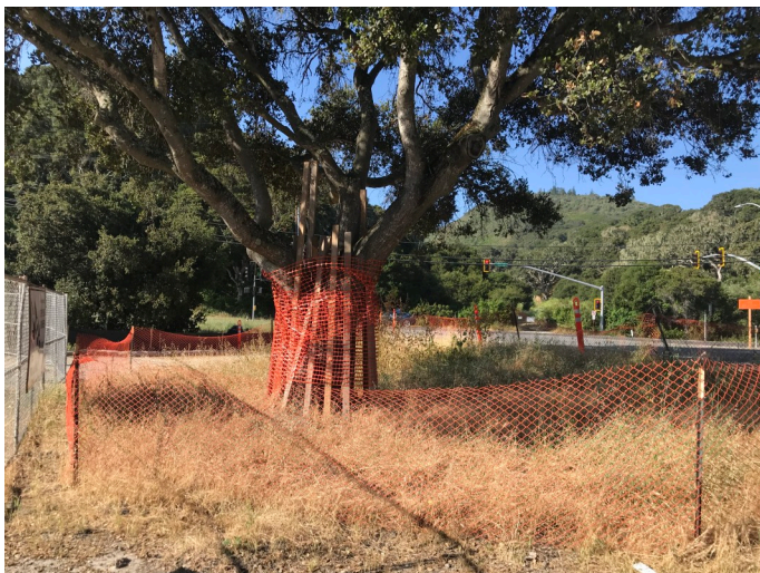
Existing tree protection adjacent to the MPE staging area at the corner of Highway 68 and York Road
