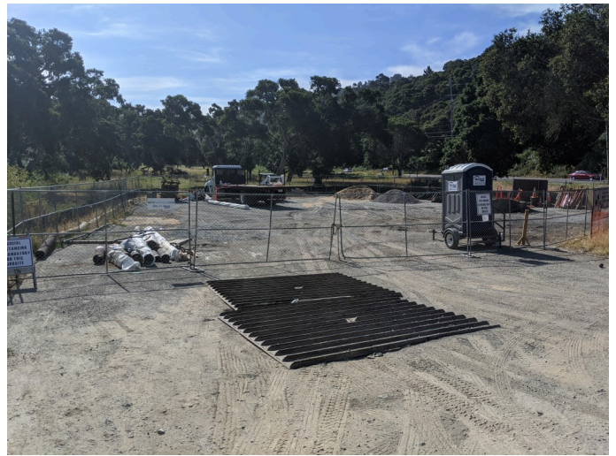
Staging area gate locked and no construction activities observed during monitoring period.
