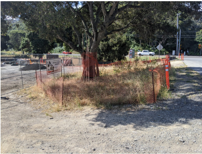
Intact ESA fencing surrounding protected oak tree adjacent to survey area.
