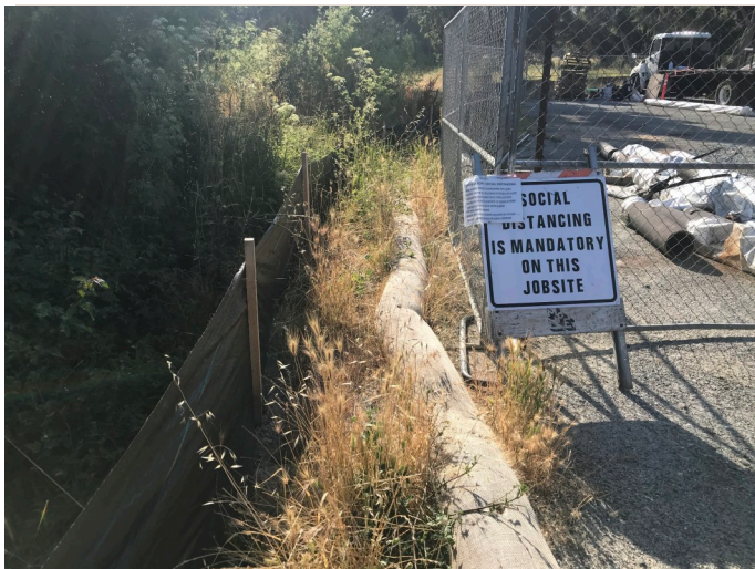
Existing silt fence surrounding the MPE staging area at the corner of Highway 68 and York Road
