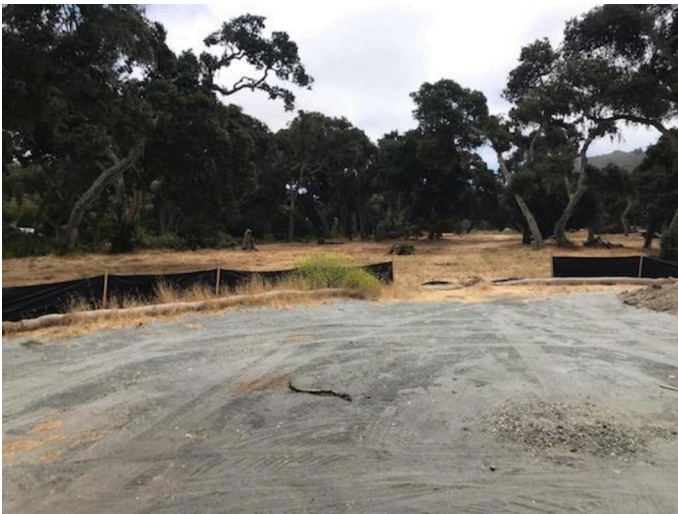
Silt fencing in need of repair at staging area.
