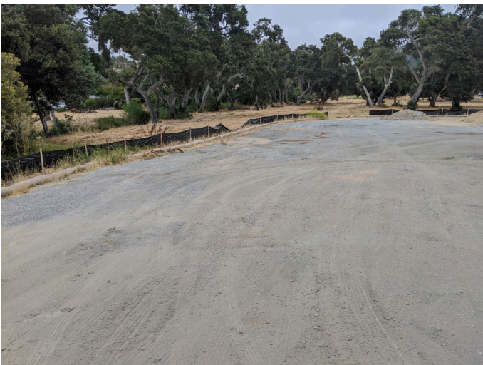
Inactive staging area, silt fencing in need of repair.
