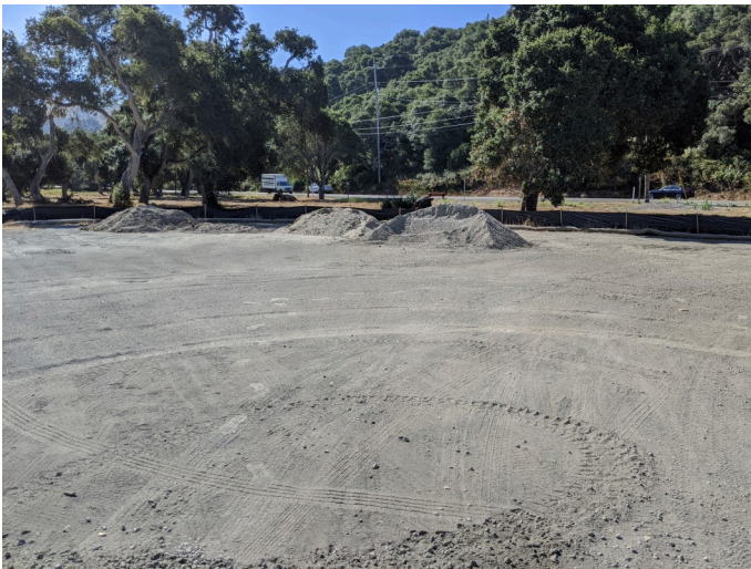
Materials storage in need of removal in staging area.
