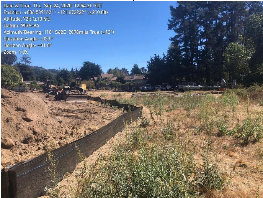
Photo 2. Vehicles parked outside of designated staging/temporary impacts zone.
