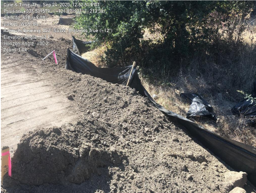
Photo 1. Silt fence in need of repair
