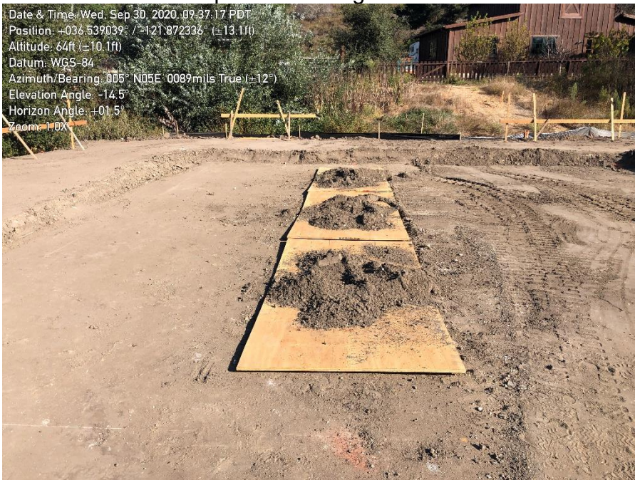
Photo 2. Excavation covered. Several gaps noted along edges.
