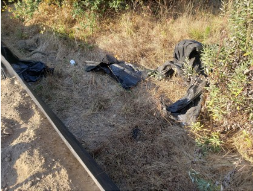
09/30/2020 - Trash located outside of exclusion fence should be collected and properly disposed of.
