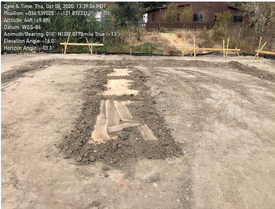
Photo 2. Carmel Valley Pump Station: Excavated area within graded pad has been adequately covered to prevent wildlife entrapment.
