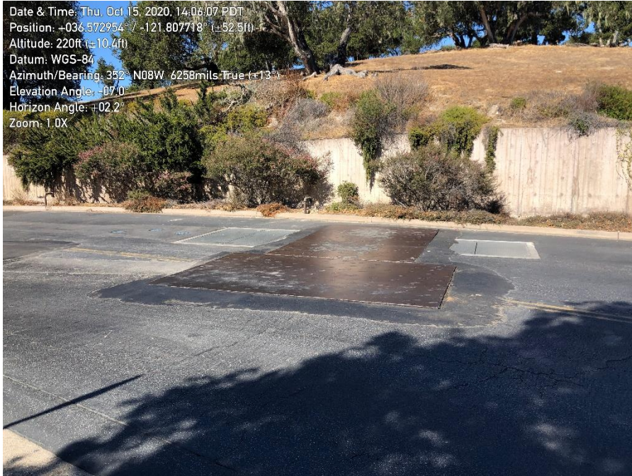
Photo 1. Ryan Ranch – Bishop Interconnection Improvements: Location of scheduled work on Blue Larkspur Lane.
