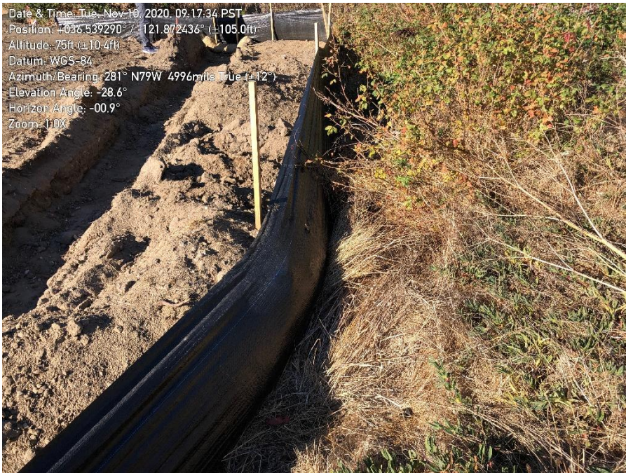
Photo 1. Carmel Valley Pump Station: small section of silt fence compromised.
