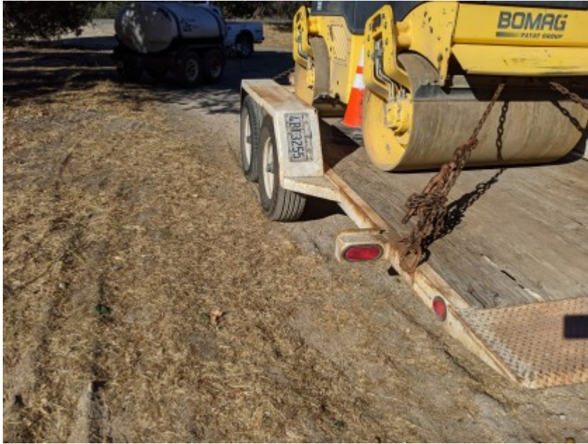
11/09/2020 - Equipment within unapproved staging area.
