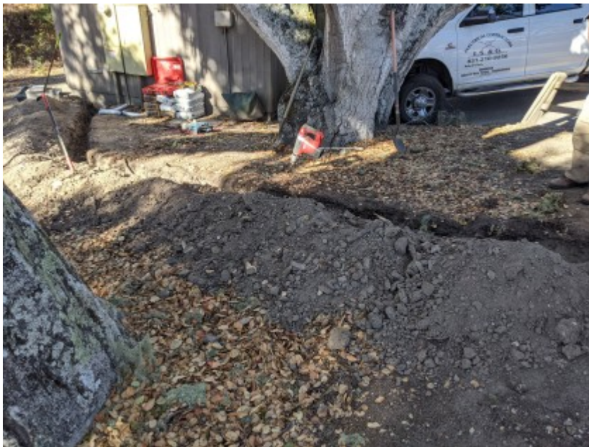
11/09/2020 - Trenching to pump station for electrical conduit adjacent to Blue Larkspur Lane.
