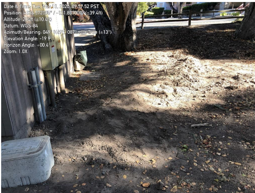
Photo 5. Ryan Ranch – Bishop Interconnection Improvements: Trenching for pump house connection complete. Installation of erosion control BMPs is recommended.
