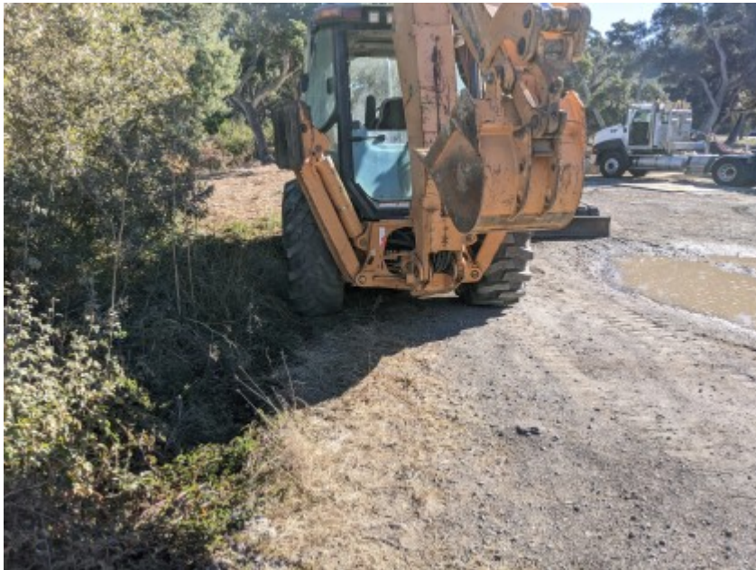
11/09/2020 - Equipment within unapproved staging area.
