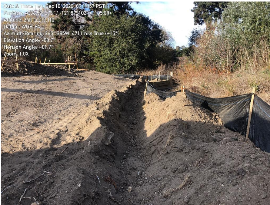
Photo 1. Silt fence near pad.
