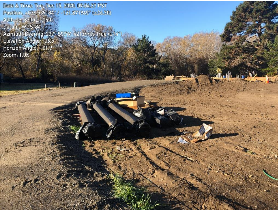
Photo 4. Pipes stored on site capped.
