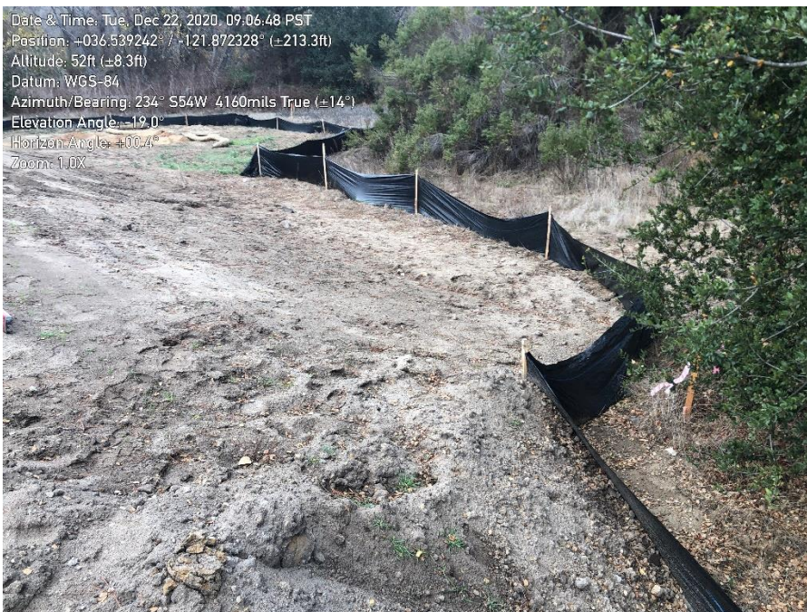
Photo 2. Silt fence at south end of site.
