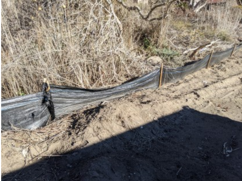
12/21/2020 - 1. Exclusionary fencing in need of repair.
