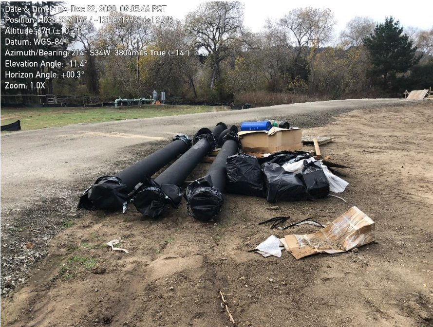
Photo 4. Pipes stored on site capped.
