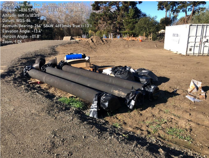
Photo 4. Pipes stored on site capped.
