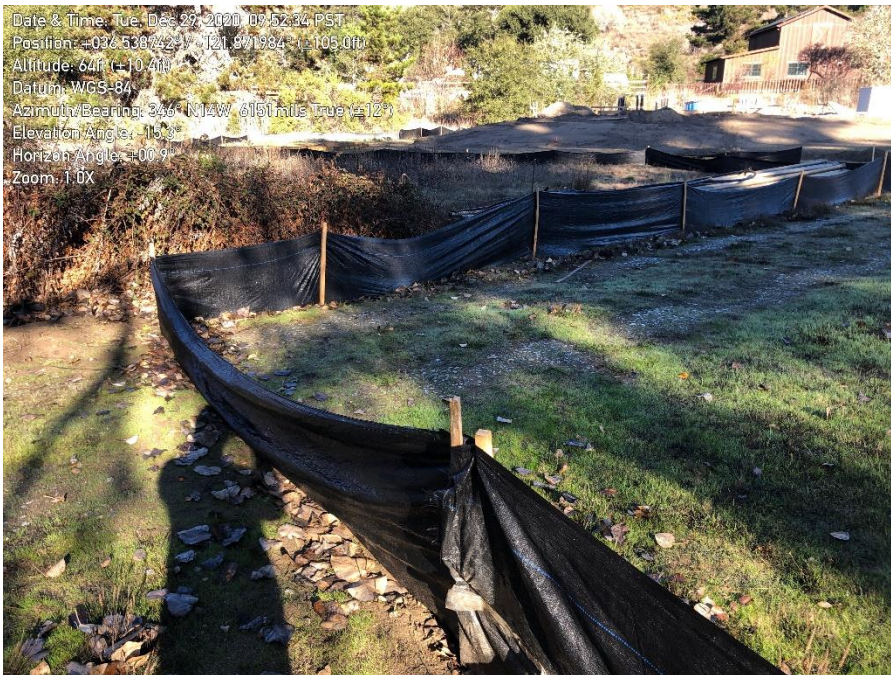
Photo 2. Silt fence at south end of site.
