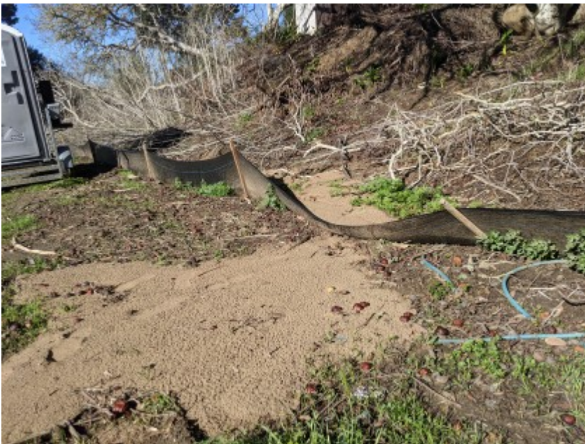
02/01/2021 - Section of exclusionary fencing damaged by erosional feature.
