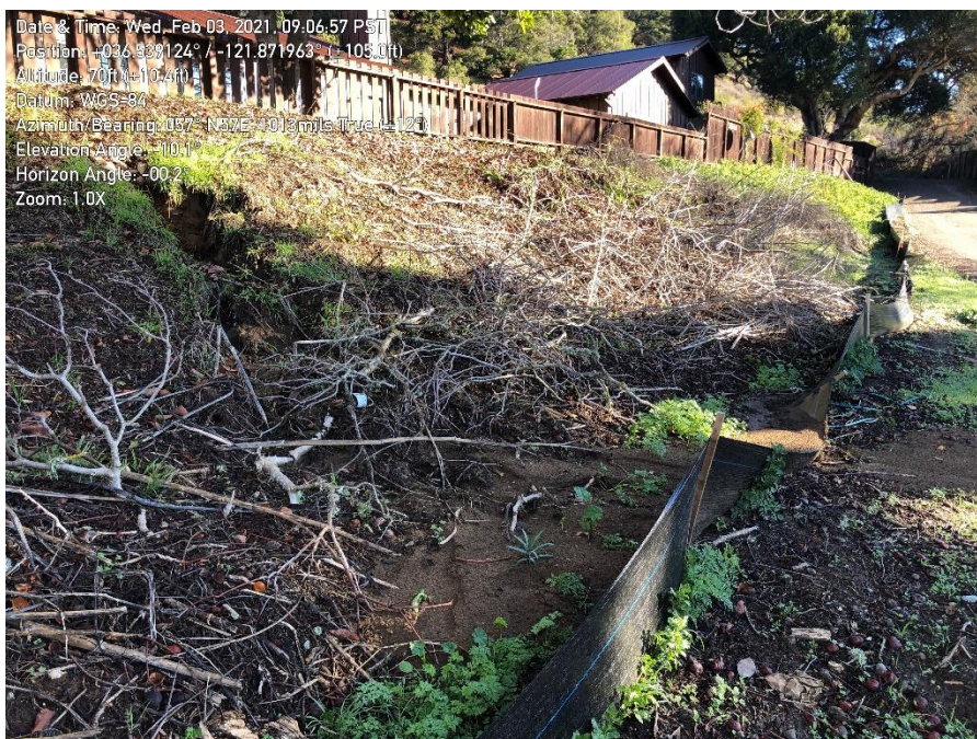
Photo 2. Silt fence compromised due to erosion.
