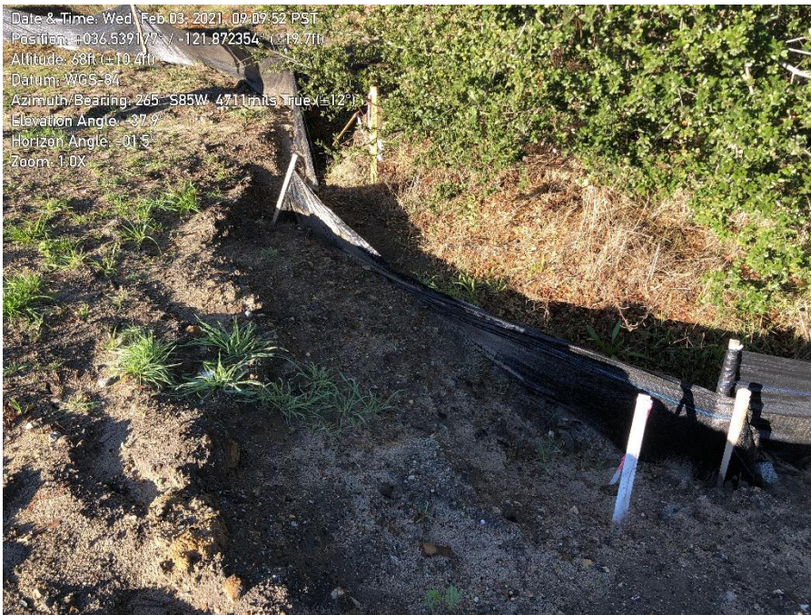
Photo 5. Silt fence down and in need of repair.
