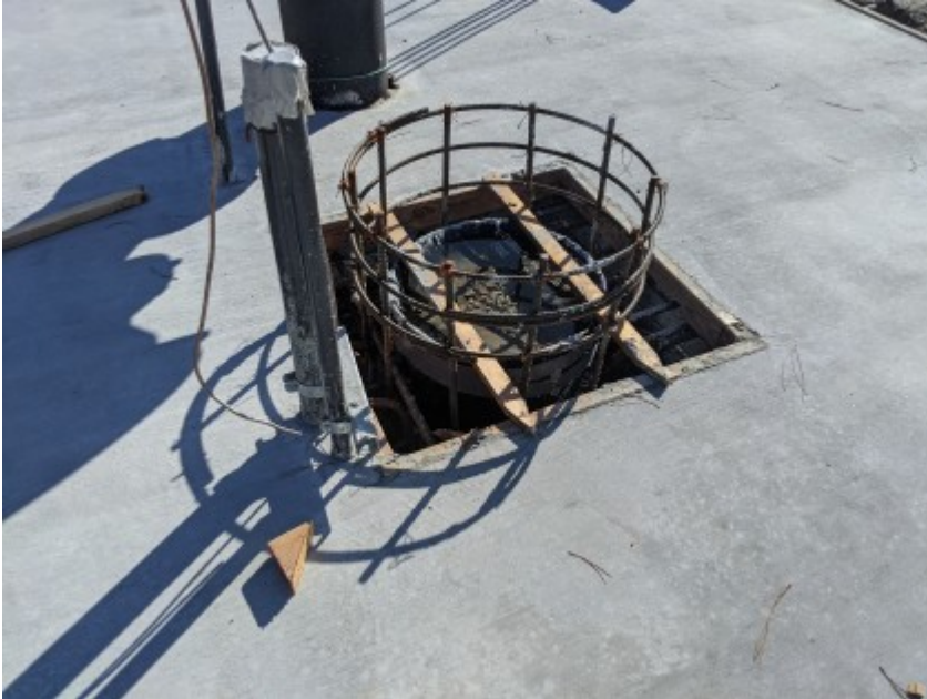
02/01/2021 - Potential pitfall trap within work area in need of protective covering.
