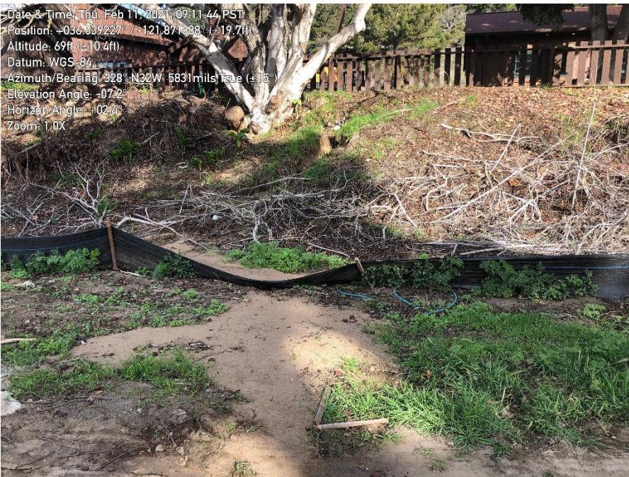
Photo 2. Silt fence compromised due to erosion.
