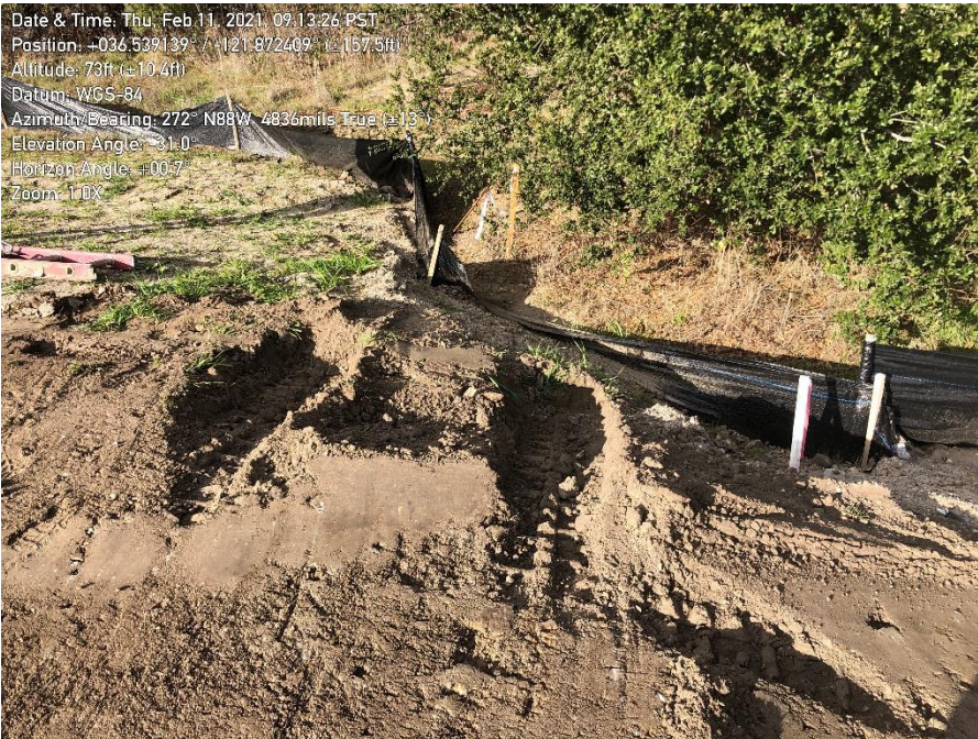
Photo 5. Silt fence down along west edge and in need of repair.
