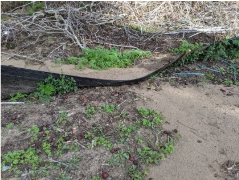
02/11/2021 - Section of exclusionary fencing damaged by erosional feature.
