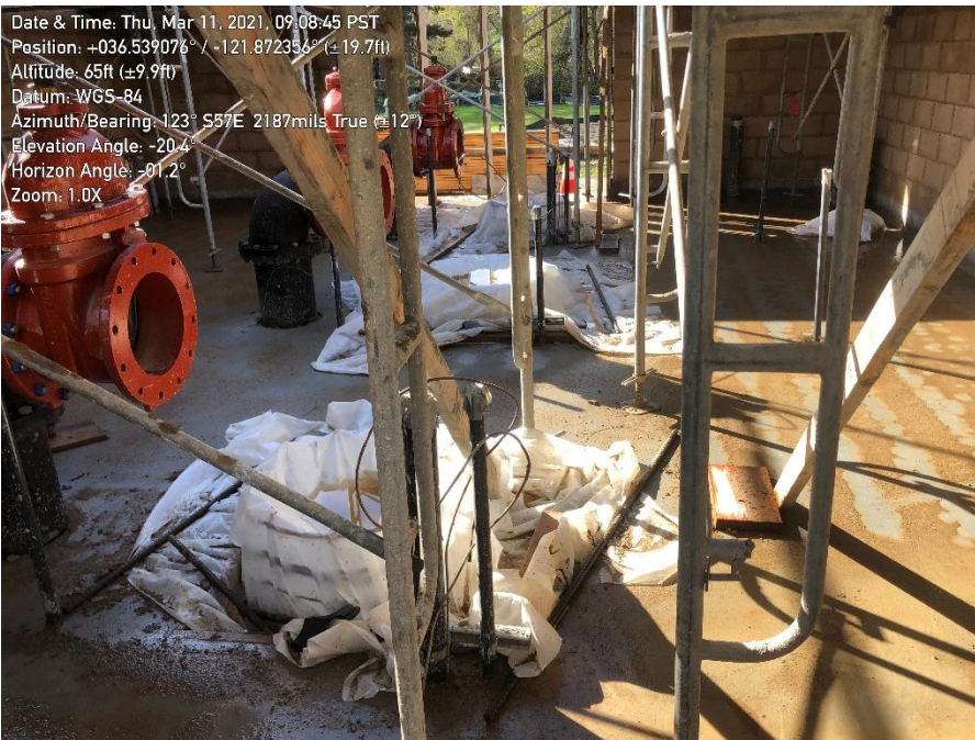
Photo 2. Interior of pump station.
