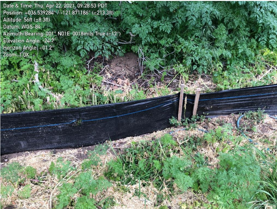
Photo 4. Tear in silt exclusion fence due to weed control activities.
