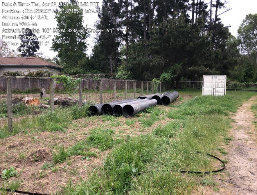
Photo 3. Uncapped pipes should be inspected prior to moving.
