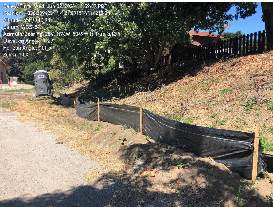
Photo 2. Exclusion fencing in acceptable condition.
