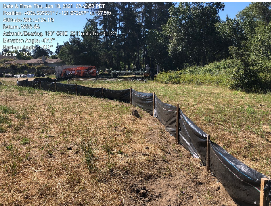
Photo 2. Exclusion fencing in acceptable condition.
