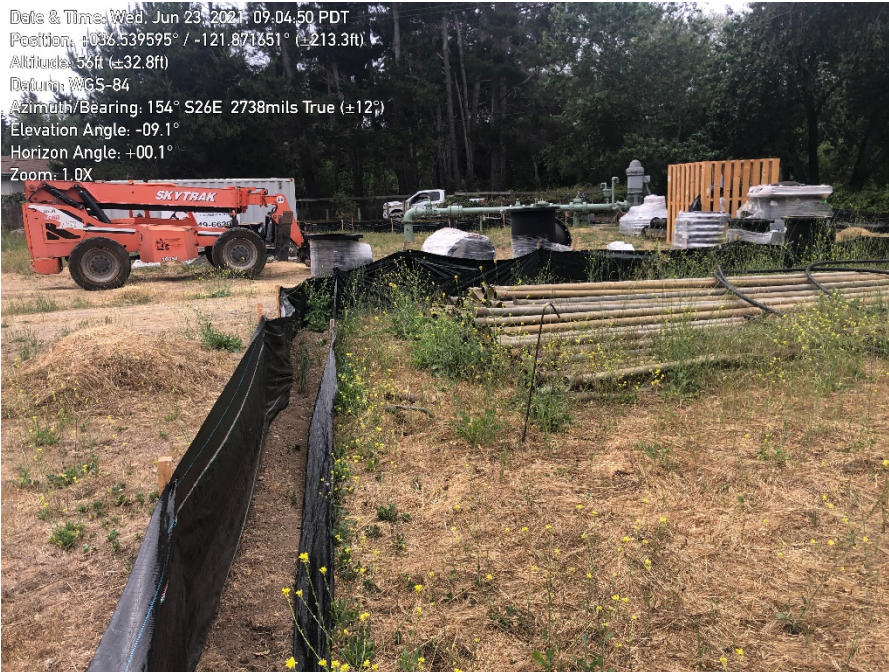
Photo 2. Exclusion fencing in acceptable condition.
