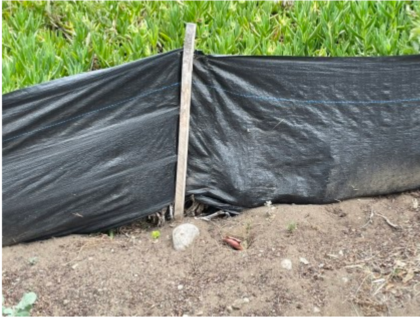
06/23/2021 - Hole in exclusion fence, fixed prior to leaving site.
