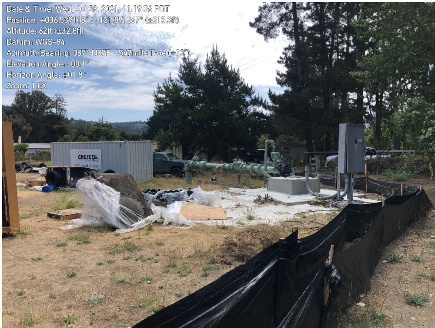
Photo 4. Old well has been filled with concrete and remains to be demolished. Pipe capped to prevent wildlife entry.
