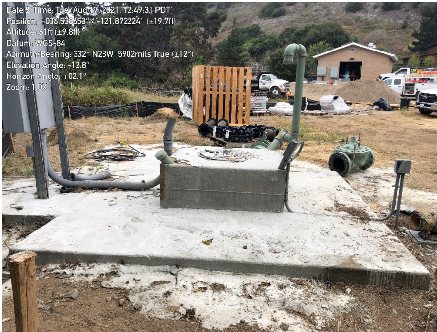
Photo 3. Excess bentonite from well closure remains on site.
