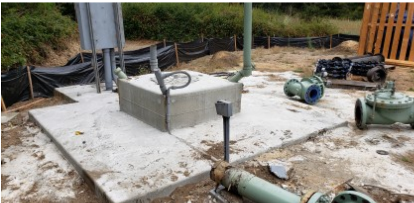
08/17/2021 - Bentonite has not been removed yet, DD&A reminded project contractor that this area needs to be cleaned prior to any precipitation events.
