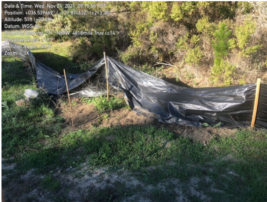
Photo 1. Silt fence not keyed-in.
