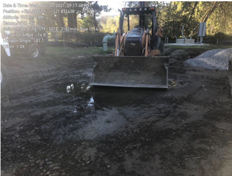
Photo 2. A large puddle has formed on site.
