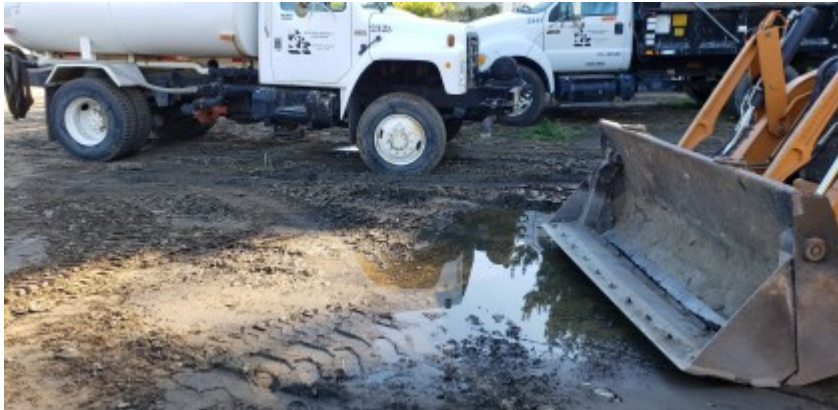
11/24/2021 - Standing water from leaking water truck. MPE to remove truck, repair leak, or discharge water before end of day.
