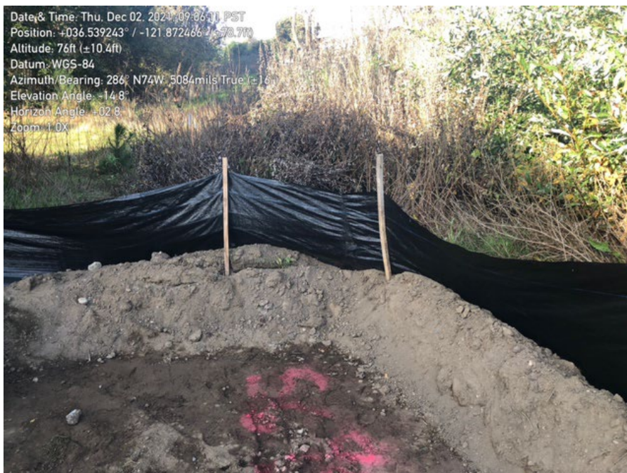
Photo 2. Damaged/downed sections of silt fence have been reinstalled.
