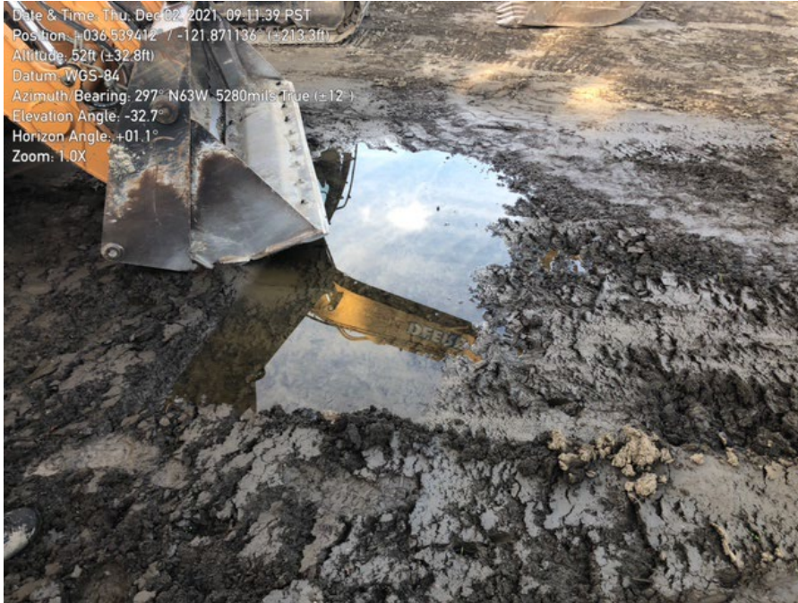
Photo 3. Puddle from leaking water truck. Water truck leak has been repaired.
