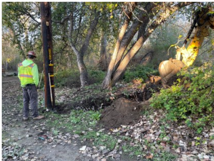
12/08/2021 - Broken waterline outside of silt fencing being contained.
