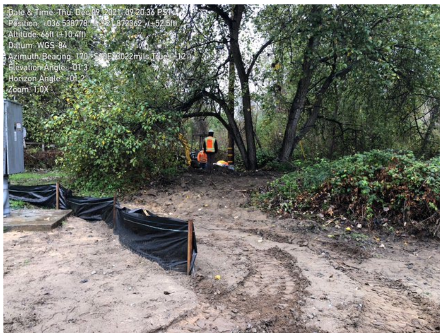
Photo 4. Location of electrical conduit outside of fenced area.
