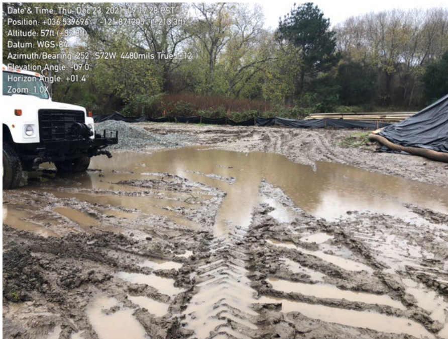
Photo 4. Ponding from recent rain events.
