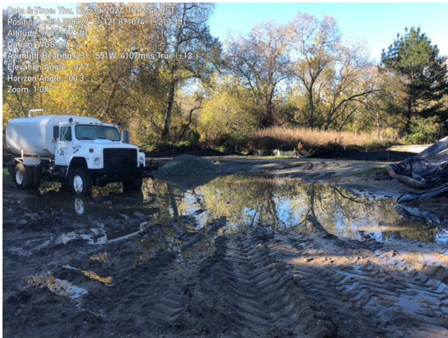
Photo 4. Ponding from recent rain events.
