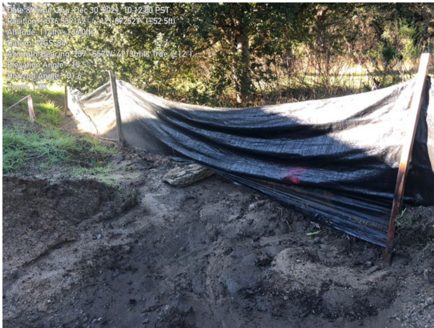
Photo 3. Gap under silt fence.
