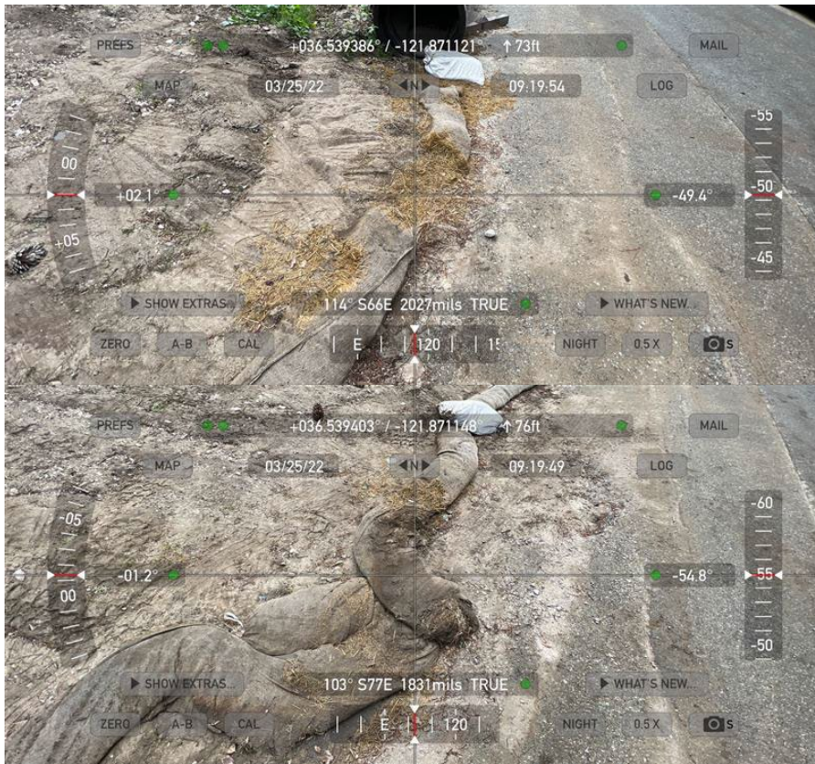
Photo 4. Straw waddles deteriorating
