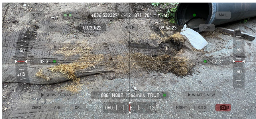
Photo 4. Straw waddles deteriorating
