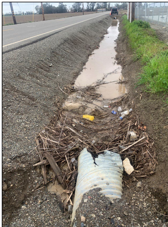
Photograph 4: Culvert 2 and Ditch 2b along north side of Project Area. Debris and trash observed at culvert opening. East aspect. 3/22/23
