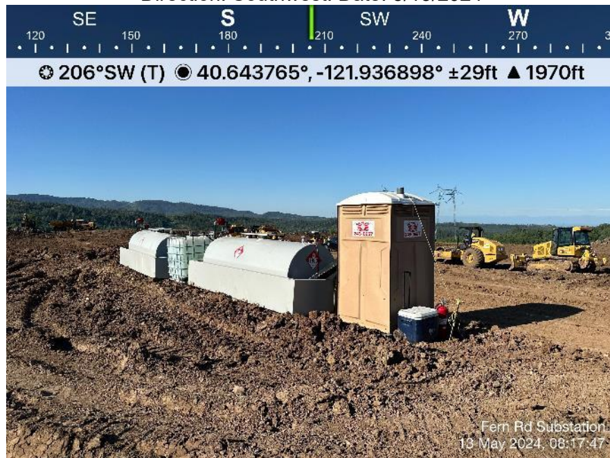
Photo 14. View of fuel tanks, DEF tank, and porta-potty located in substation area. Direction: Southwest. Date: 5/13/2024
