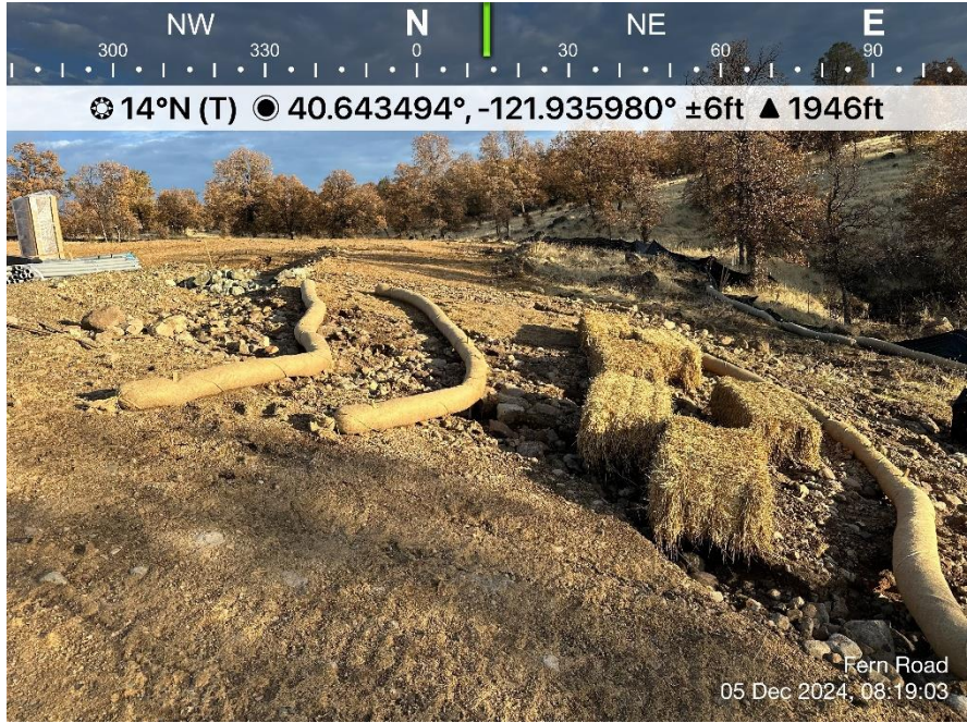
Photo 17. View of slope erosion at northeast corner of substation pad. Direction: North. Date: 12/5/2024
