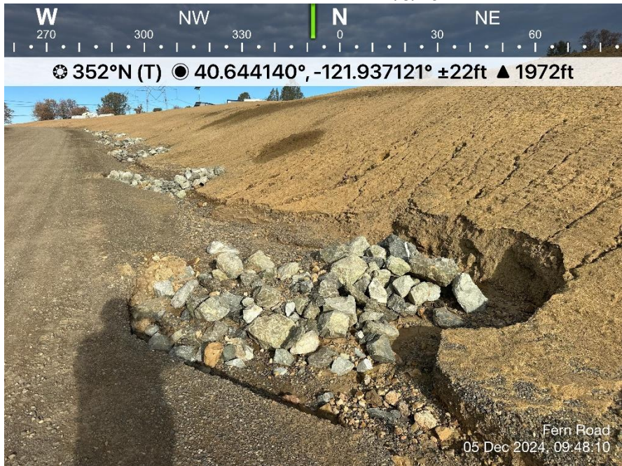
Photo 18. View of slope and road erosion along access road swale check dams. Direction: North. Date: 12/5/2024
