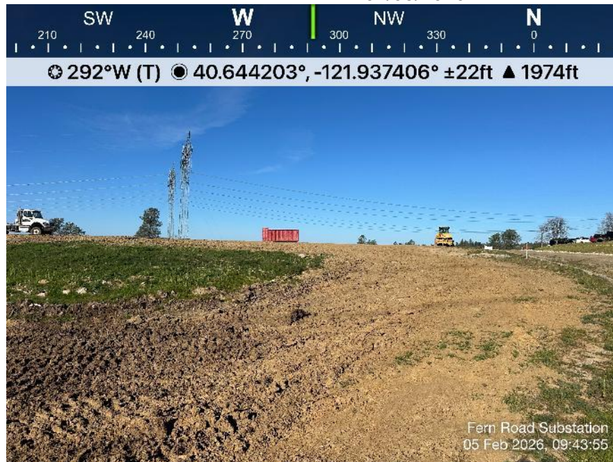
Photo 21. View of bare area west of access road last used by PG&E that needs stabilization. Direction: West. Date: 02/05/2026
