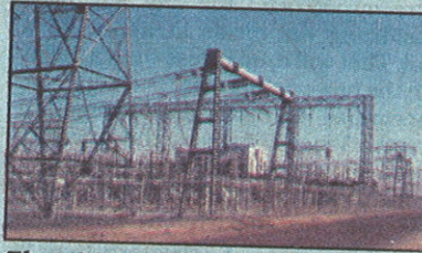
The SCE Rector substation in southeast Visalia is the destination of the power lines the power company wants to bring into the county.
