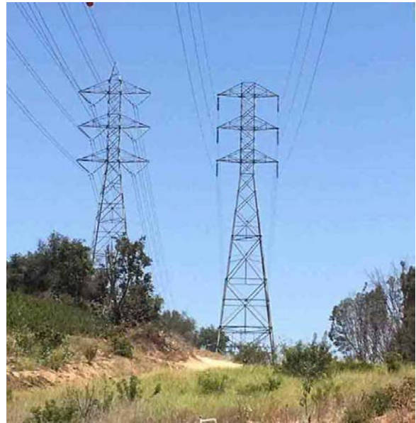
Tower Loc. 100 at right, looking north from Bresa de Loma Drive near Harmony Grove Street
