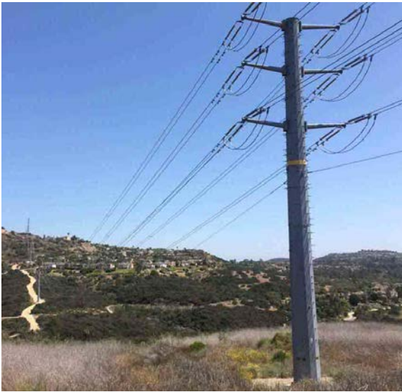
TL 13811/13825 pole looking south from W. San Marcos Boulevard
