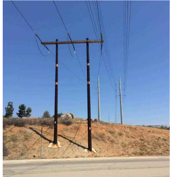
Steel H-frame tower looking north from S. Andreasen Drive; steel poles at rear
