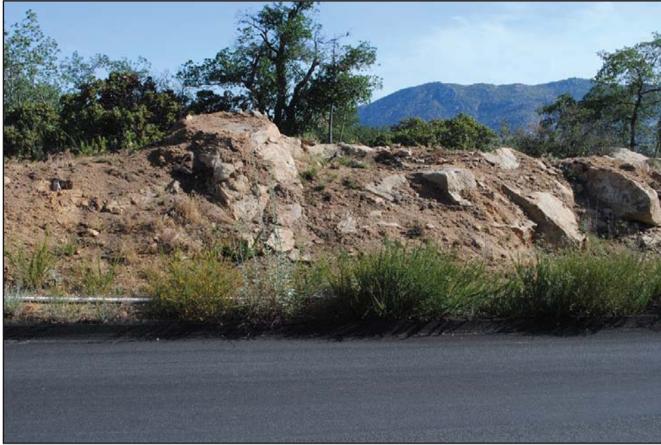
Figure 13. Site CA-SDI-20166, Overview of Outcrop Impacted by Road Construction, View to the North
