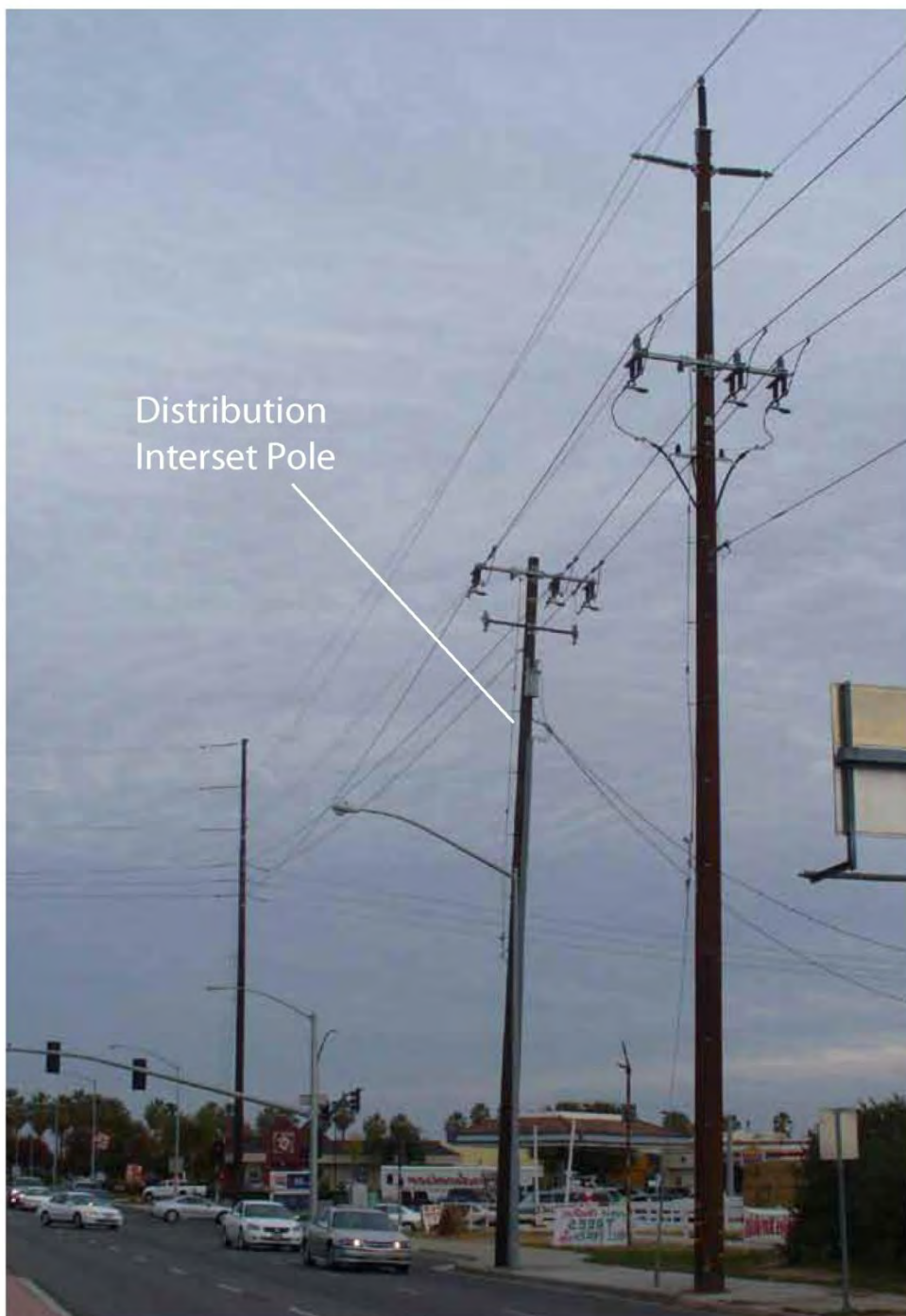
Figure 2.4-37: Typical “Topped” Wood Pole
