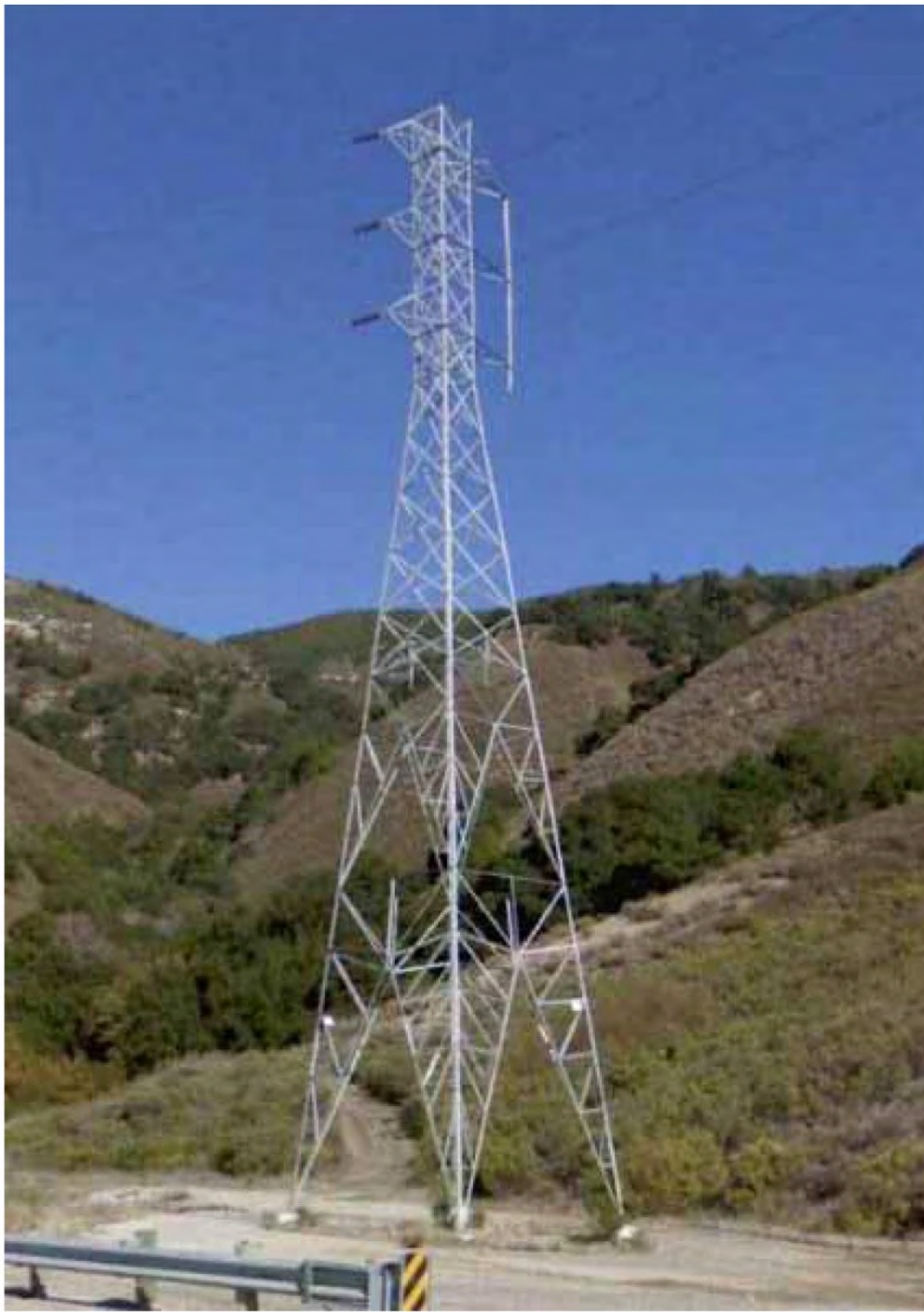
Figure 2.4-38: Typical Lattice Steel Tower
