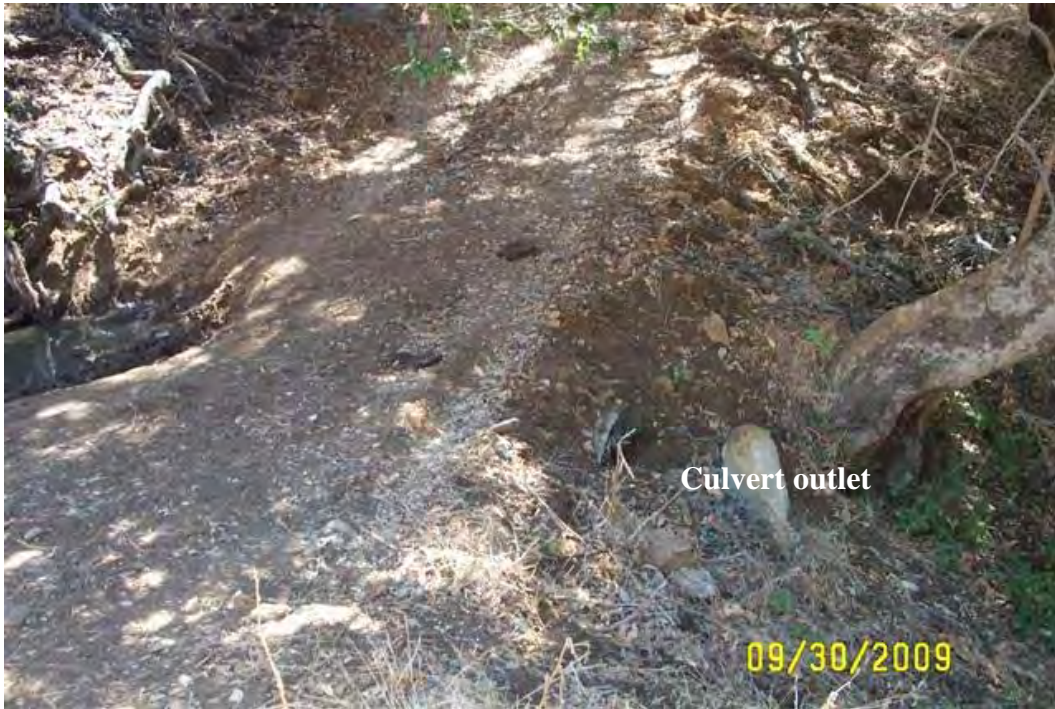
S9: Tributary to Santa Margarita Creek (NRPW), crossing along access road to Tower 69/0, culvert outlet
