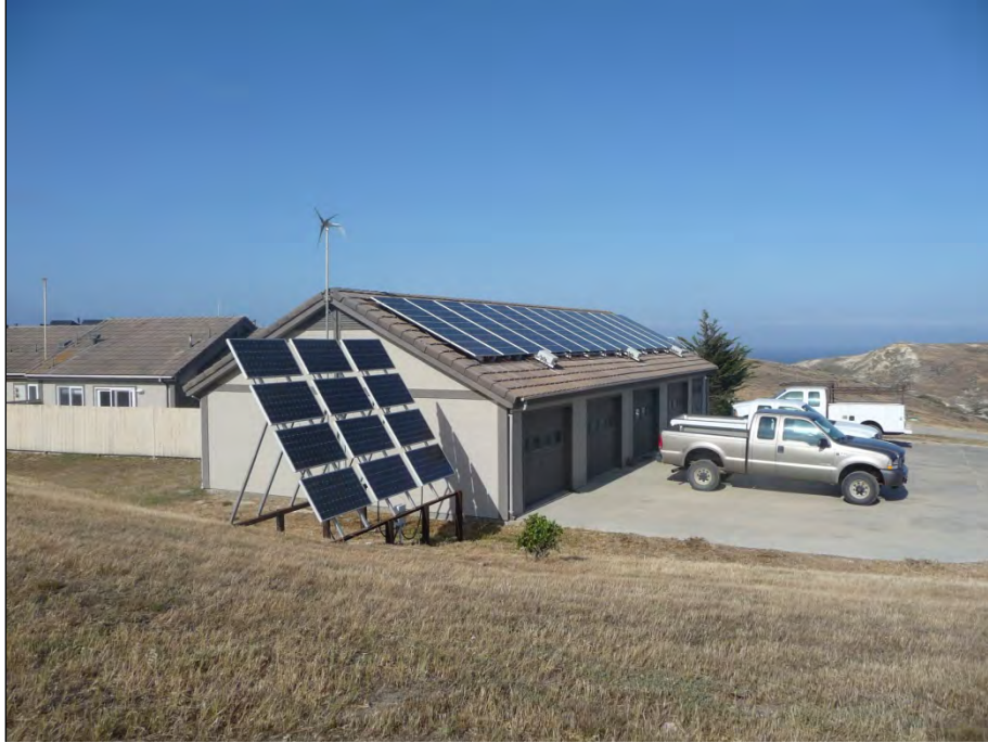
Exhibit 20. Proposed installation site for the payphone, mounted on the garage building wall next to the solar panel array. View facing east toward Main Ranch cluster, located along the shoreline and not visible from Focused APE #16. (JRP Historical Consulting, LLC)
