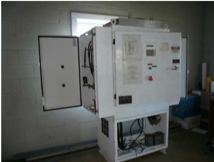
Figure 15 – battery bank and controller inside power station building
