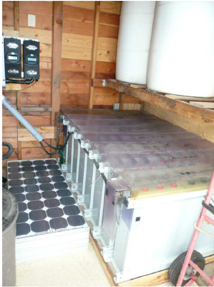
Figure 7 – Battery Bank at San Miguel Ranger Station
