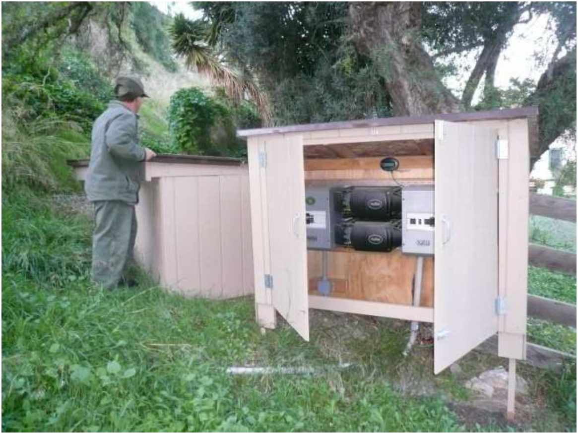
Figure 28 A – solar panel and housing at Scorpion Adobe
