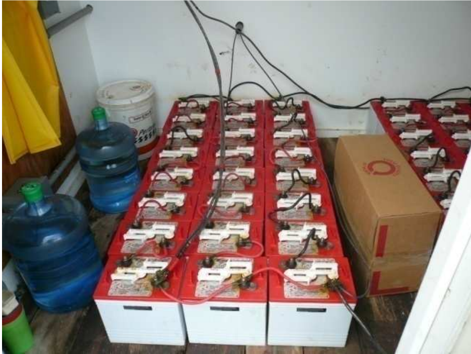
Figure 2 – Santa Barbara Ranger Station existing battery bank (3600Watts) Lat 33°28'49.70"N Long 119° 1'46.08"W
