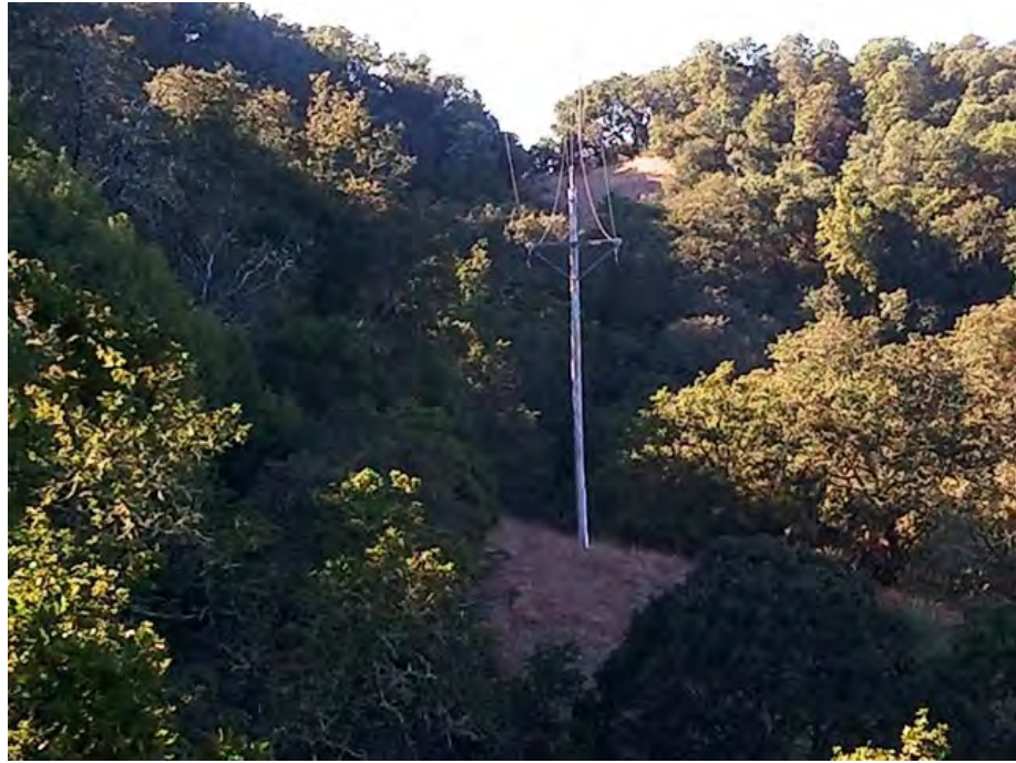
Canyon span at pole 46
