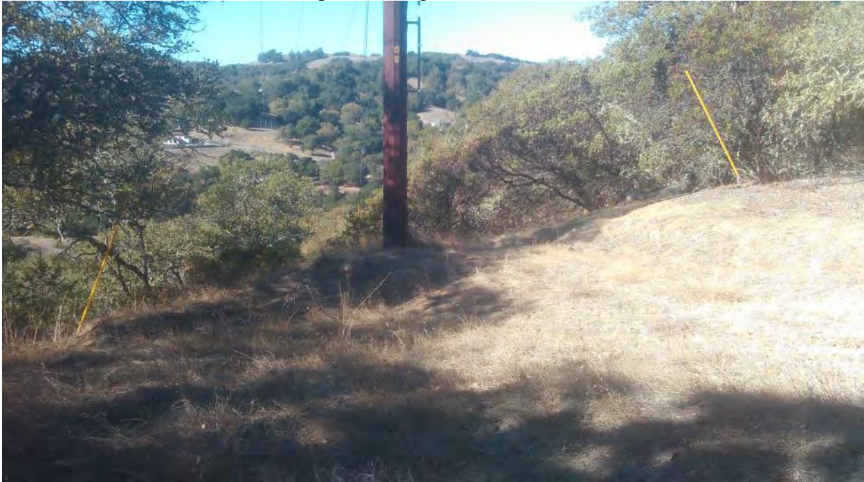
FFW14/15 – PS10; Pole 62; SW3 (photo facing north)
