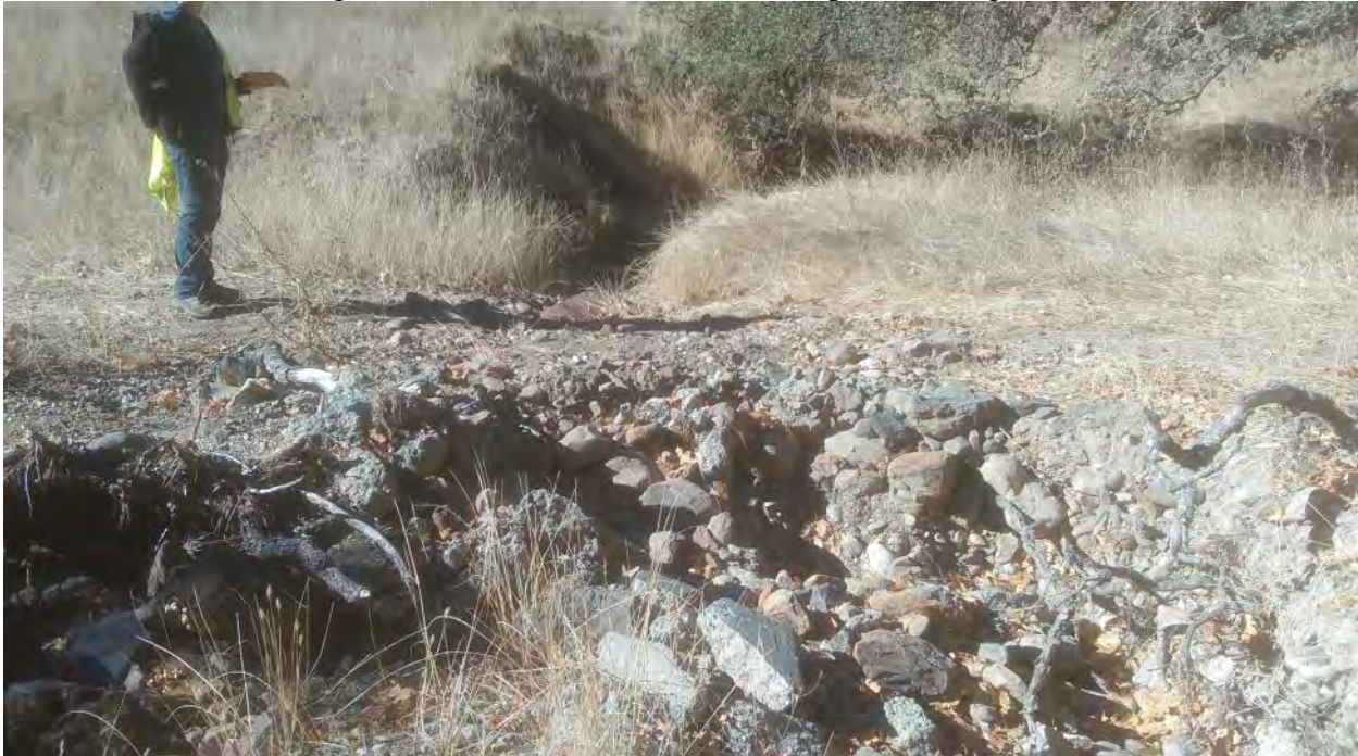
FFX8 – SEW2; Existing culvert is filled in with sediment (photo facing west)
