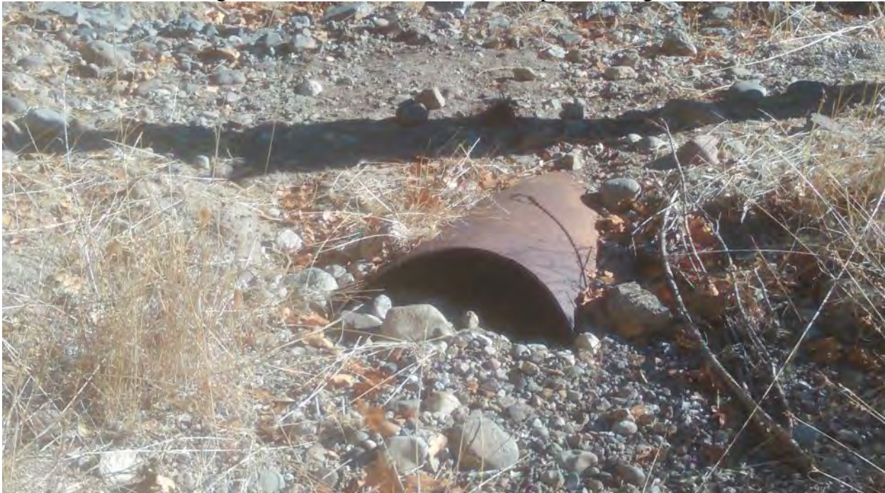
FFX8 – SEW2; Existing culvert is filled in with sediment (photo facing west)
