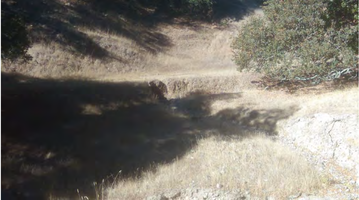
FFX9 – SEW2; Bank of adjacent watercourse eroding into road (photo facing west)
