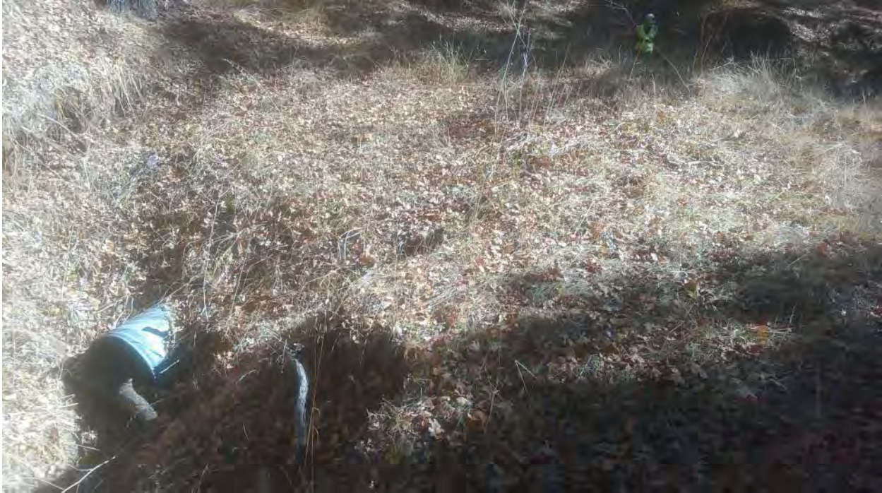
FFX15 – SEW8; Culvert crossing through bermed earth at the bottom of the drainage (photo facing west)
