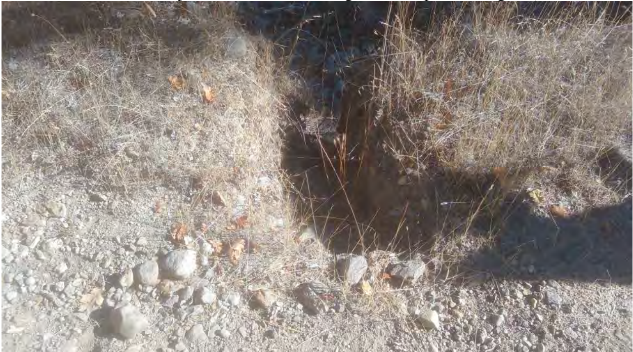
FFX9 – SEW2; Bank of adjacent watercourse eroding into road (photo facing east)
