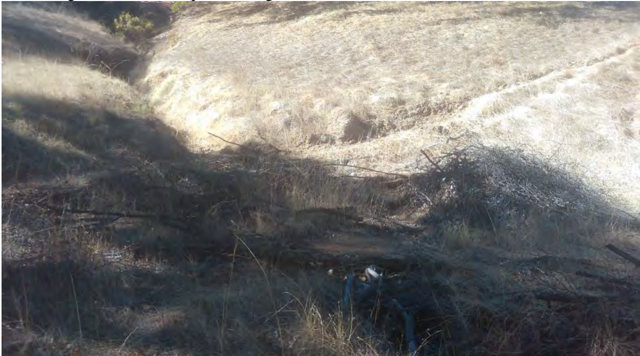
FFX14 – SEW8; Overland access route has multiple stacks of cut brush piled along the roadway, obstructing vehicular travel (photo facing north)
