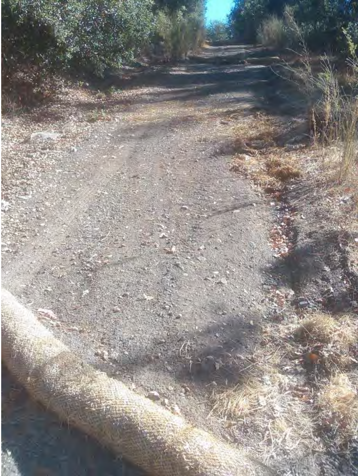
FFX1 – SEW44; Access road with seasonal surface flow and wattles (photo facing west)
