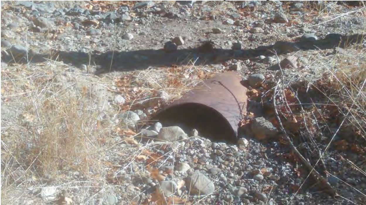
FFX8 – SEW2; Existing culvert is filled in with sediment (photo facing west)
