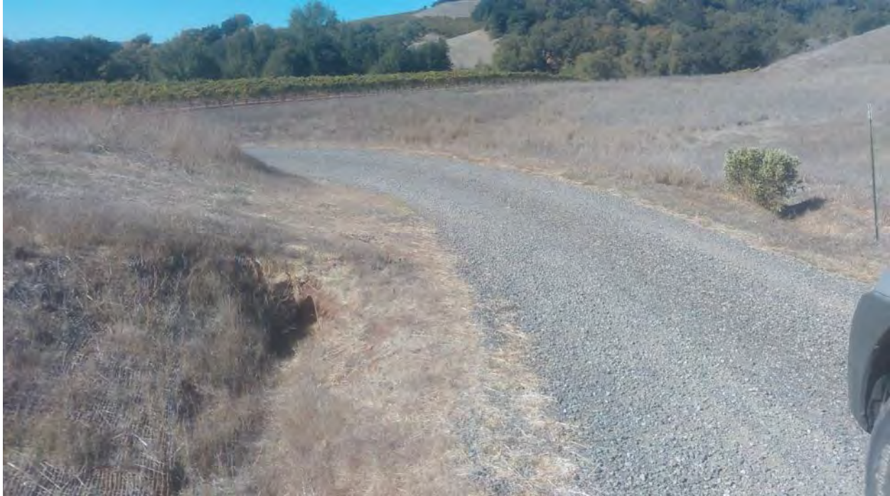
FFX17 – D5; Culvert crossing for drainage ditch under improved road (photo facing northwest)
