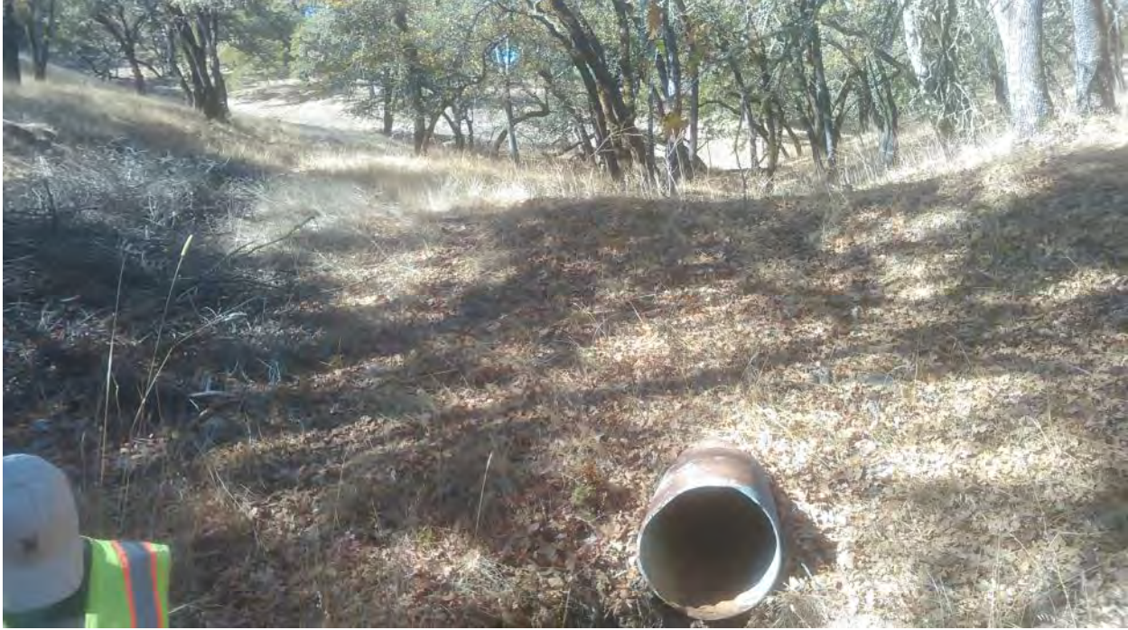
FFX15 – SEW8; Culvert crossing through bermed earth at the bottom of the drainage (photo facing north)
