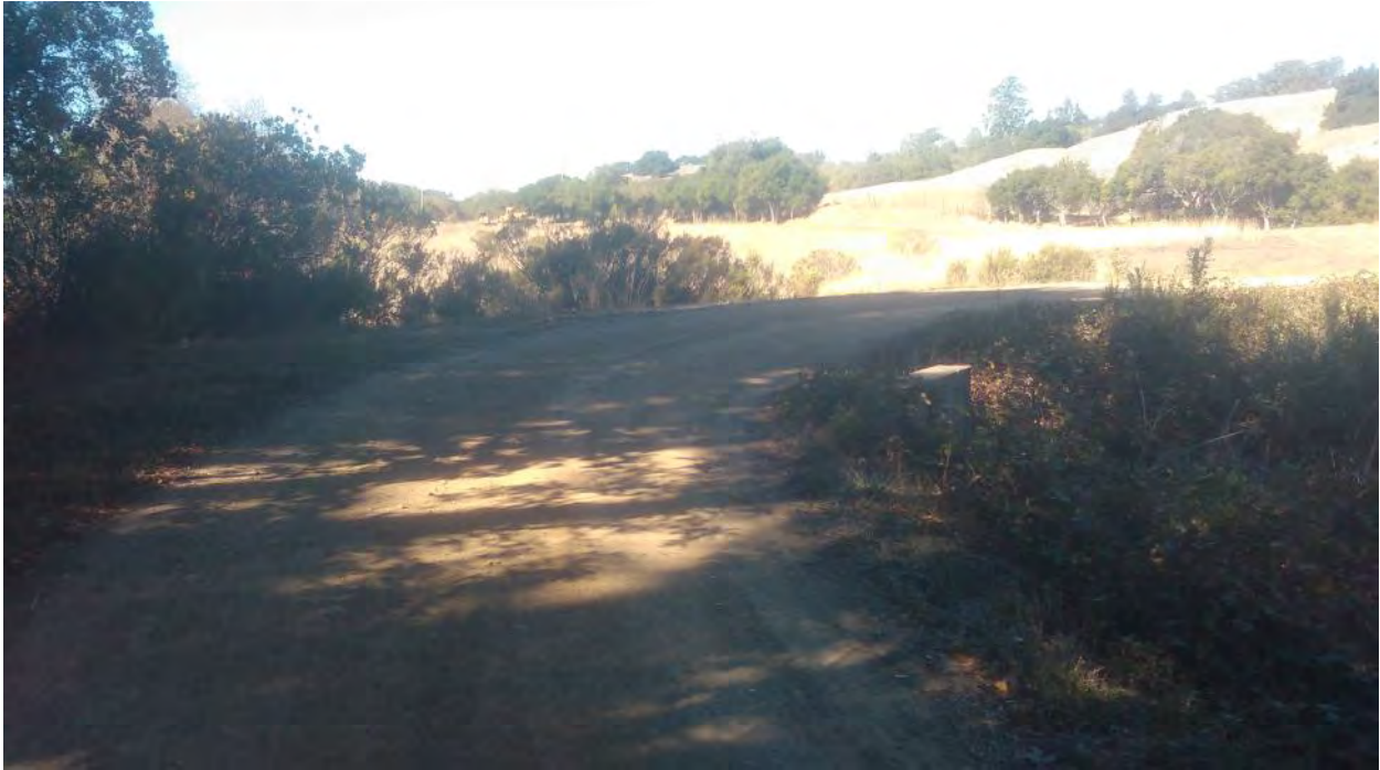
FFX13 – RIWO10; Culvert crossing occurs immediately downstream of perennial pond (photo facing northwest)
