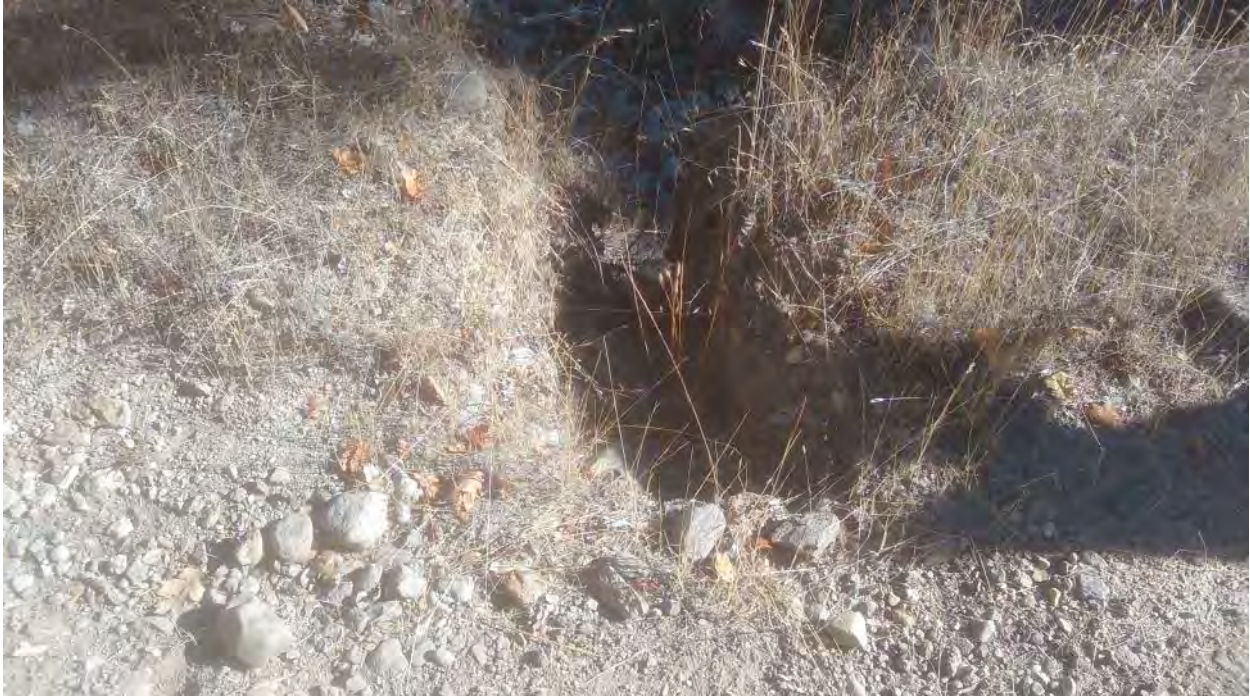
FFX9 – SEW2; Bank of adjacent watercourse eroding into road (photo facing east)
