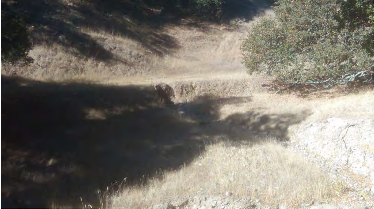
FFX9 – SEW2; Bank of adjacent watercourse eroding into road (photo facing west)
