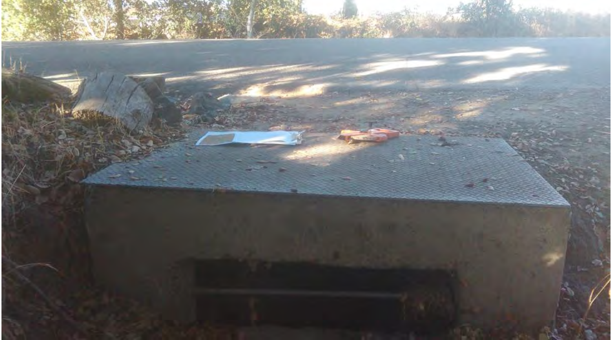
FFW1 – Pole 20; SEW41 Culvert at terminus of drainage (photo facing west)
