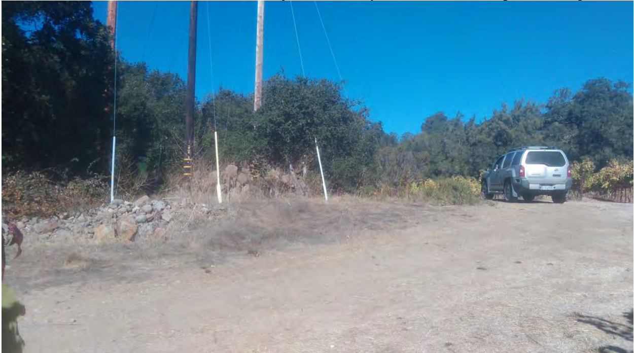
FFW18 – Pole 71; RIWO10; Work area adjacent to vineyard and woodland (photo facing north)
