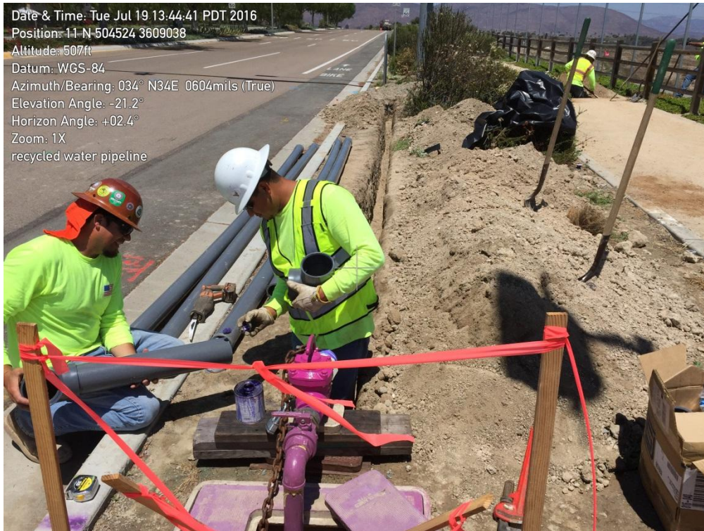
Recycled water line (07/19/16)
