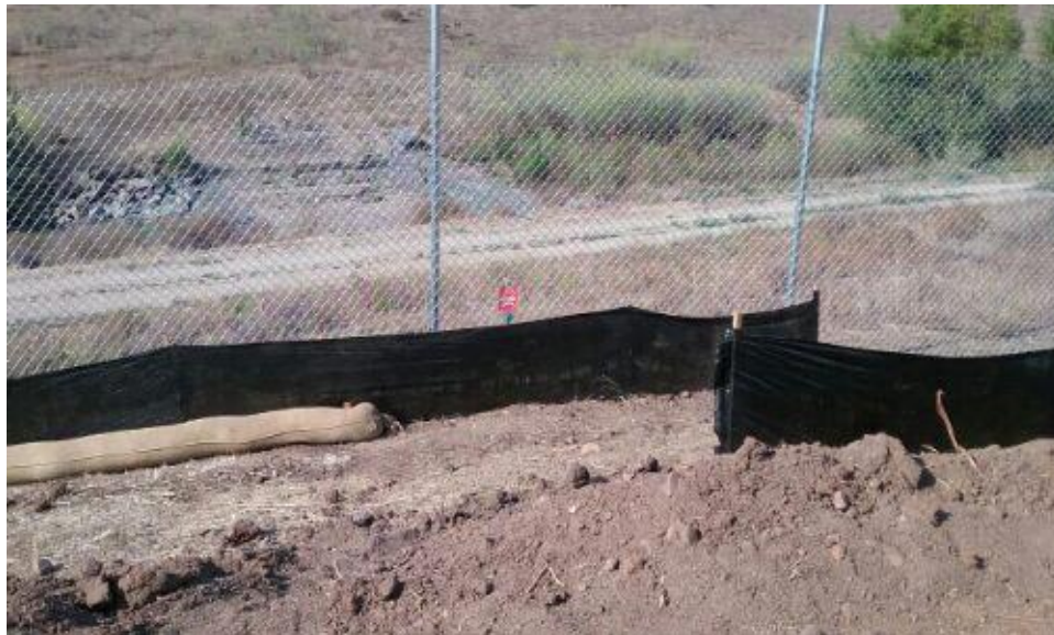
Caption Silt fencing at toe of slope and bird buffer signage. Photo Attributes~ Capture Date/Time: Fri Jul 29 2016 08:55:12 GMT-0700 (PDT) Coordinates: 32.612094, -116.95266 View Direction: South
