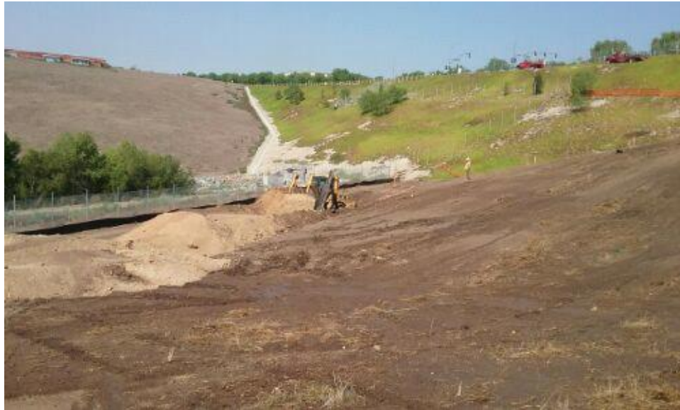
Caption Excavation for geotech investigation of toe of slope materials. Photo Attributes~ Capture Date/Time: Fri Jul 29 2016 09:34:26 GMT-0700 (PDT) Coordinates: 32.618891, -116.949731 View Direction: Southeast
