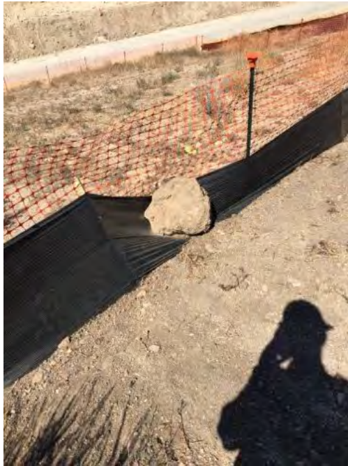
Caption Silt fence damage
