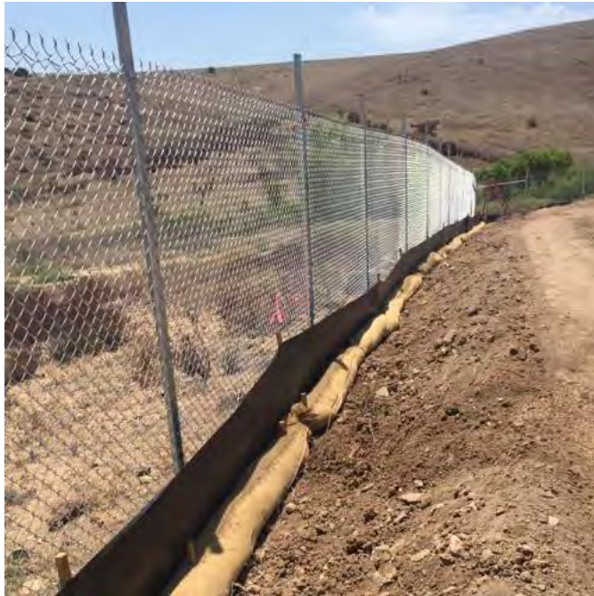
Caption Silt fencing and straw wattles along sw slope Photo Attributes~ Capture Date/Time: Wed Aug 03 2016 12:28:54 GMT-0700 (PDT) Coordinates: 32.618434, -116.948441 View Direction: Southwest
