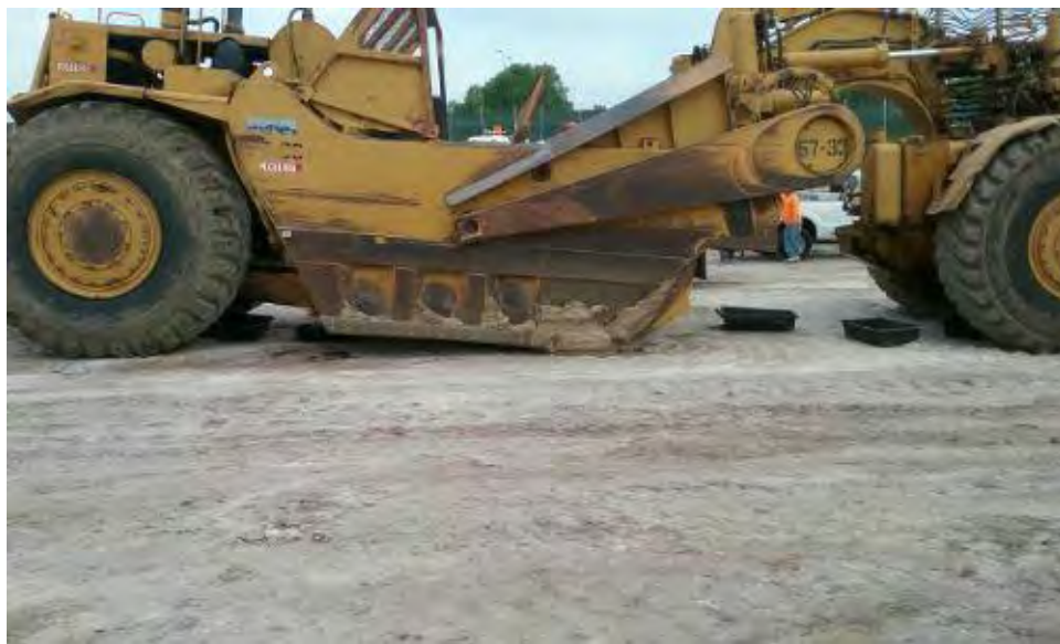
Caption Proper spill prevention provided beneath equipment over night.
