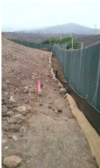
Caption Silt fence intact despite rocks rolling downhill along southern limit.
