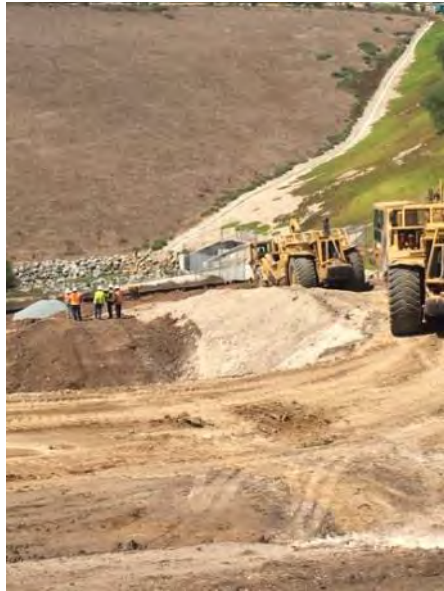
Caption Grading equipment and monitors Photo Attributes~ Capture Date/Time: Tue Aug 02 2016 13:13:15 GMT-0700 (PDT) Coordinates: 32.617928, -116.953040 View Direction: West
