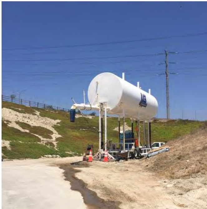
Caption Upper water tank leaking
