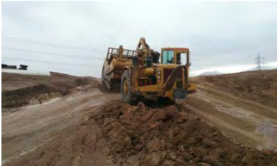
Caption Caterpillar D9s did not start until 8 am to allow placement of sub-drains before grading continues.
