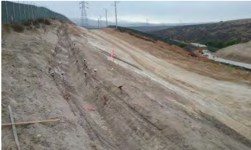
Caption Drainage ditch, slope, and finished grade of access road on north end.
