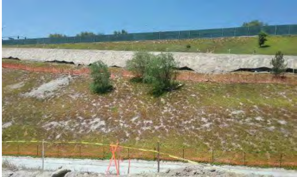
Caption Fallen silt fence next to excavation on west part of site.
