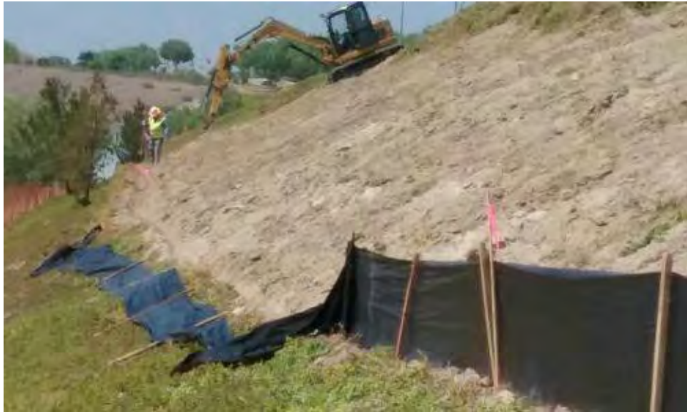
Caption Vegetation removal and silt fence installation for access road widening on west part of site.
