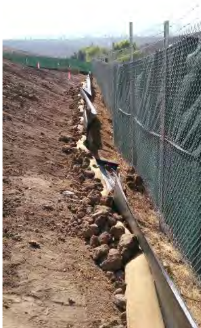
Caption Damage to silt fence on south part of site.
