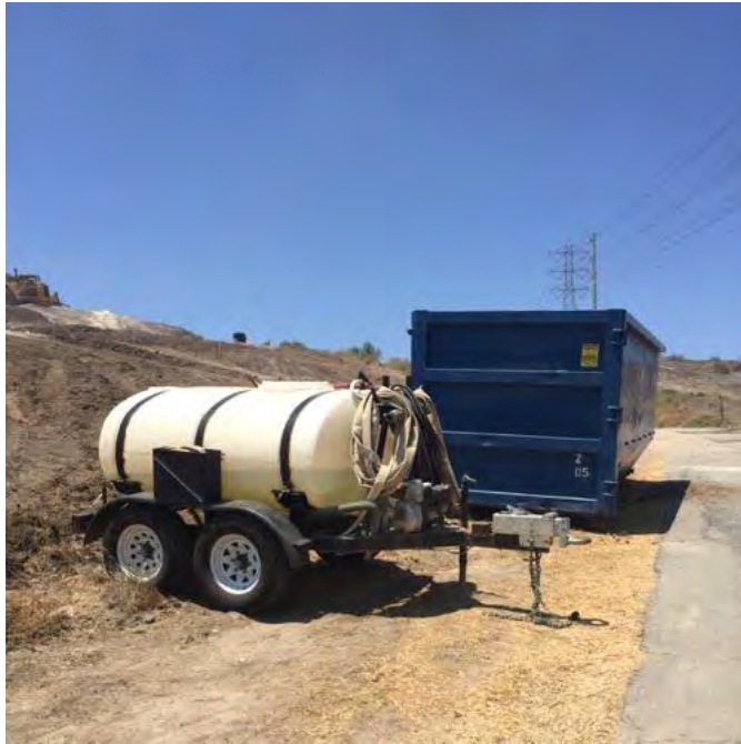
Caption Third water tank on site next to dumpster
