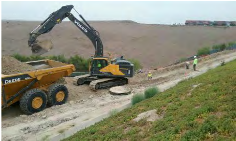
Caption Soil excavation for access road retention wall on west part 'of site.
