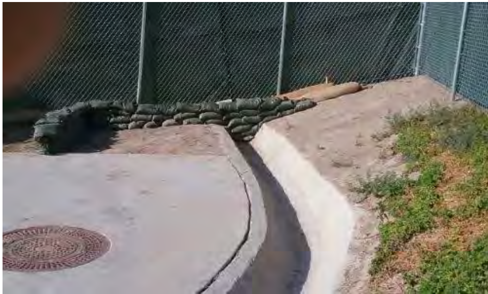
Caption Additional gravel bags to reinforce sediment control BMPs at bottom of concrete V-ditch.
