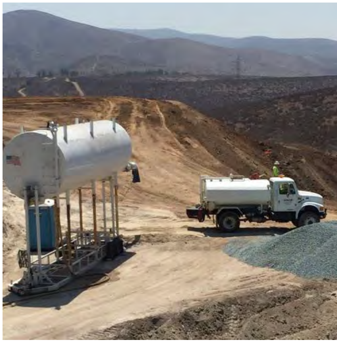
Caption Low site water tank
