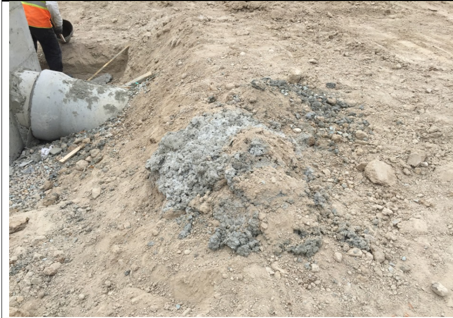
Photograph 1: On September 19, 2016 construction debris (concrete) was observed spilled on to the ground.
