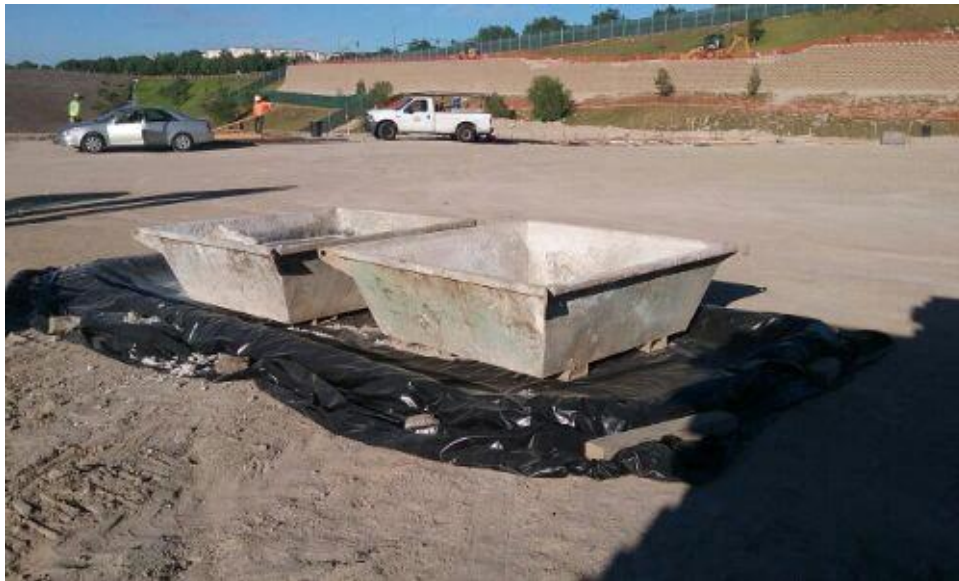
Caption Concrete washouts on visqueen liner.
