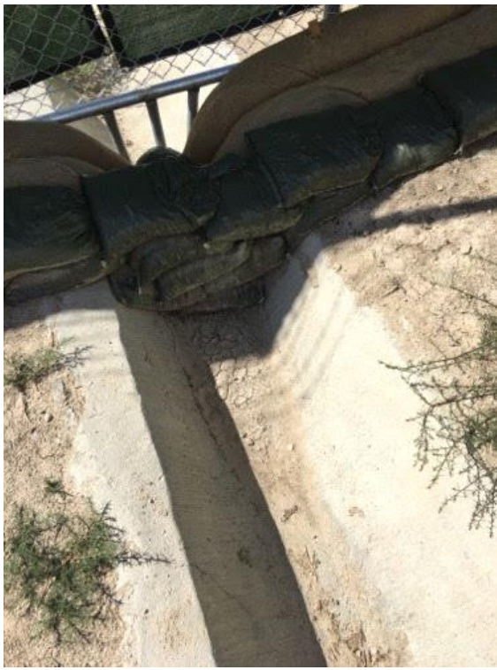
Caption Sand bags within brow ditch with dirt trapped onsite
