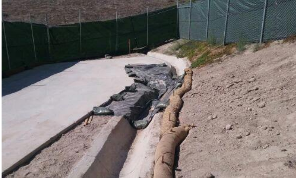
Caption Visqueen lining lower parts of brow ditch at NW corner of site.
