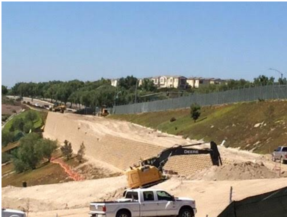
Caption Verdura wall and excavating storm drain on NW side of project site
