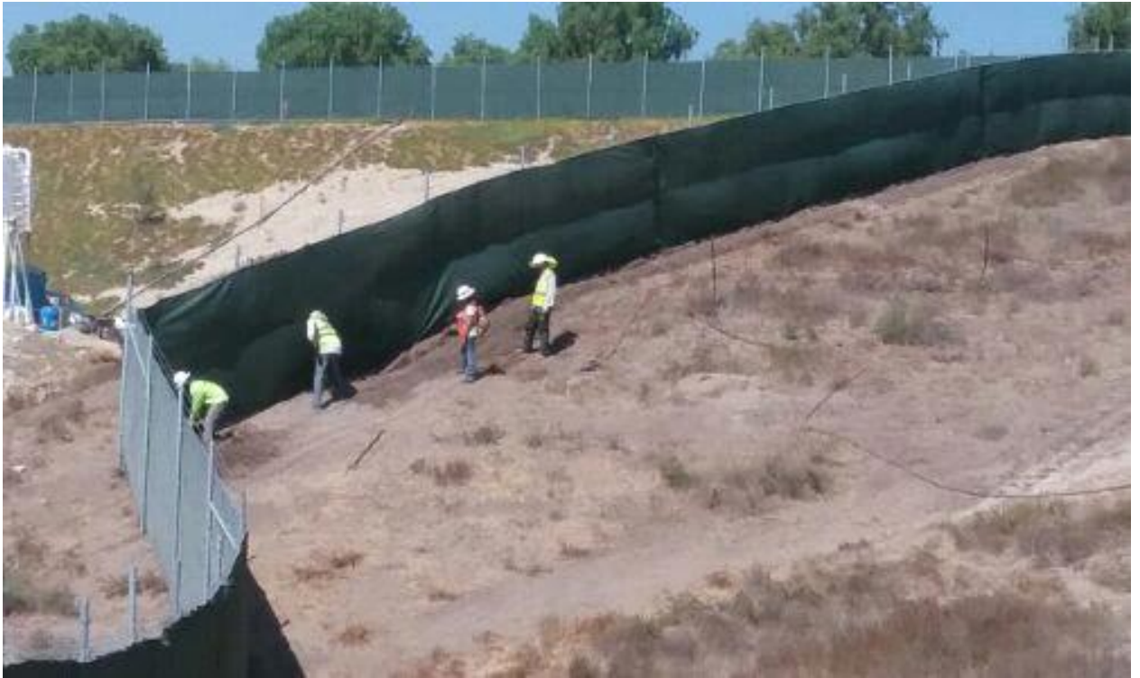
Caption Digging for grounding wire, outside fence but within LOI, cultural and Native American monitors present.
