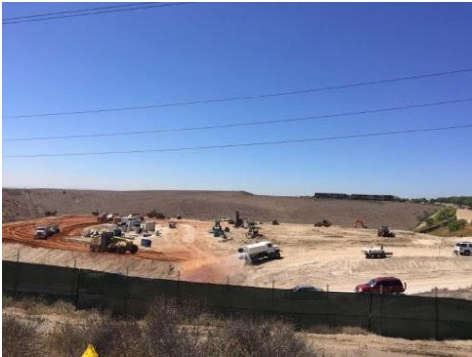
Caption Substation pad site with water truck. Red dirt is imported fill.
