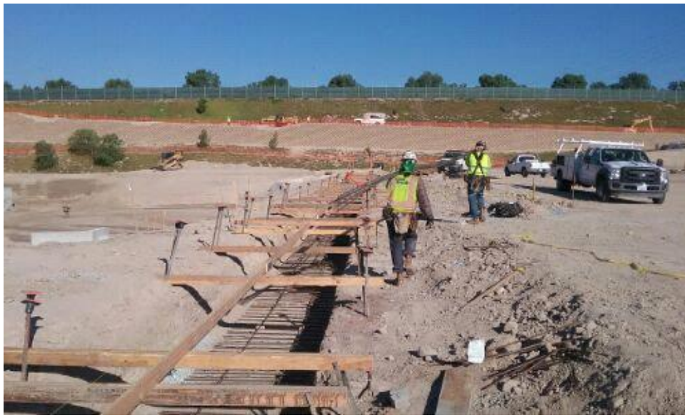
Caption Free placing rebar in trench for concrete pour for screening wall.
