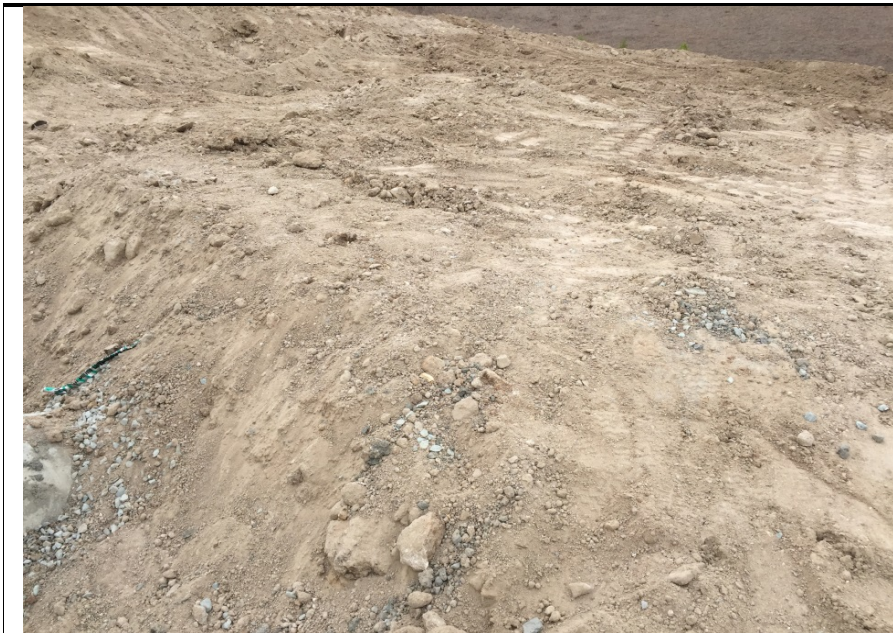
Photograph 2: On September 19, 2016 the spilled concrete was picked up and properly disposed of.
