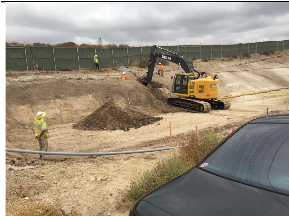
Photograph 4: Construction of project site drainage facilities occurred during the week of September 12, 2016.
