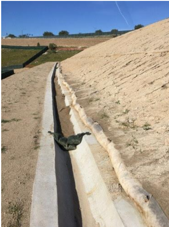
Caption Fiber roll and brow ditch need maintenance
