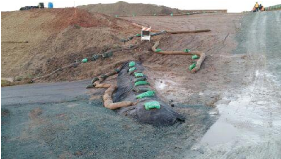
Caption Erosion control devices below most active construction road were effective in 0.25" rainfall event.
