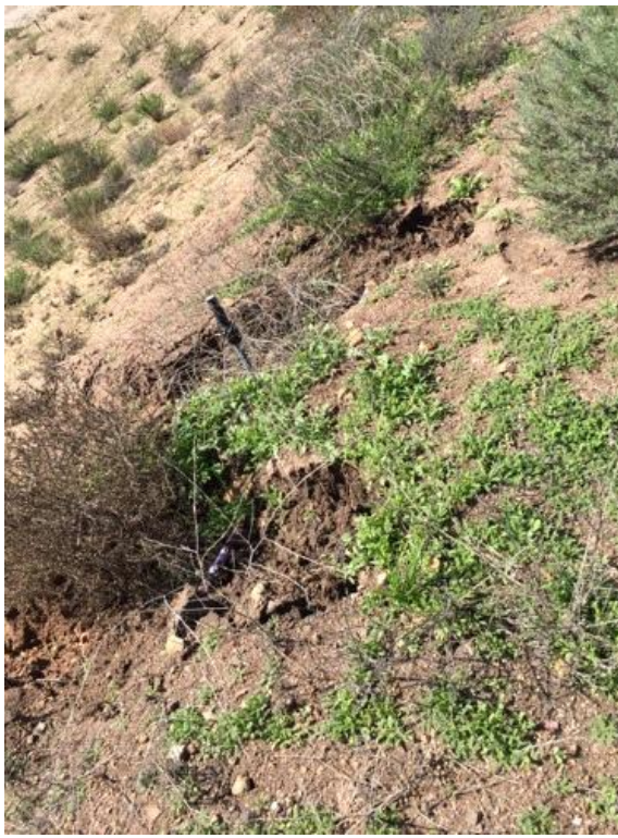
Caption Two more erosion gullies have formed from offsite flows. Photo Attributes Capture Date/Time: Wed Jan 04 2017 10:57:14 GMT-0800 (PST) Coordinates: 32.618466, -116.946787 View Direction: Northwest
