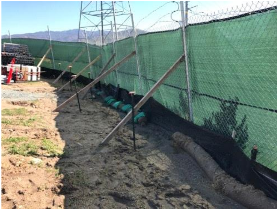
Caption Perimeter fence shored up until fence contractor can do repairs.
