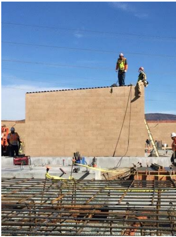
Caption Roofing for control shelter.
