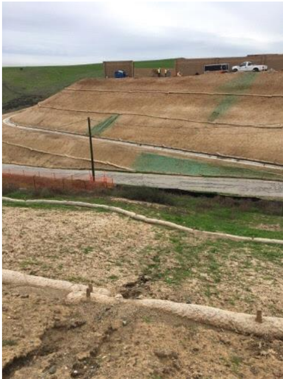
Caption Slope erosion on both slopes
