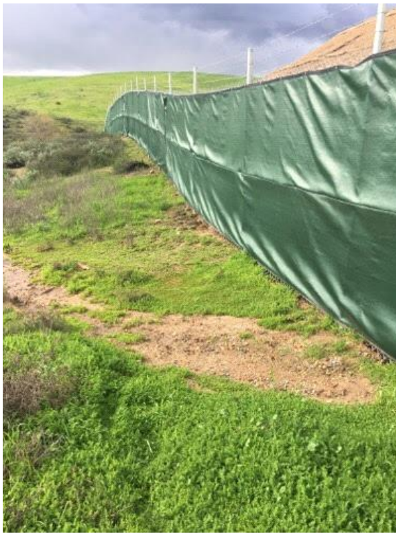
Caption Secondary outfall - flow downstream is from western-most eroded area. No surface flow at the 2ndary outfall (foreground eroded area).
