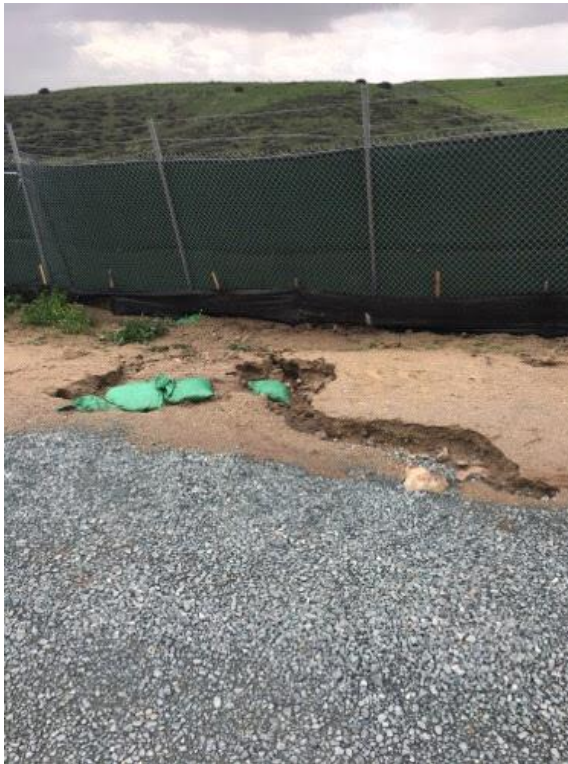
Site erosion along access road entrance
