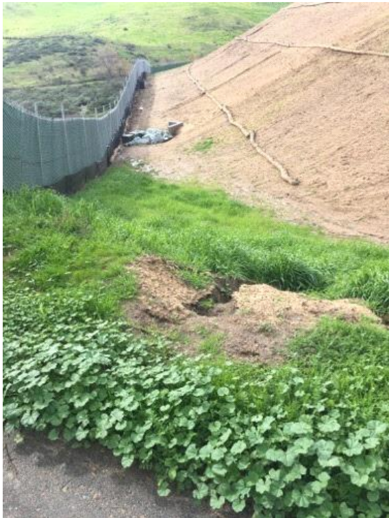
Caption Erosion on road slope below construction trailer
