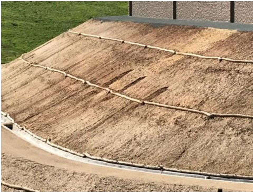
Caption Erosion on south slopes.
