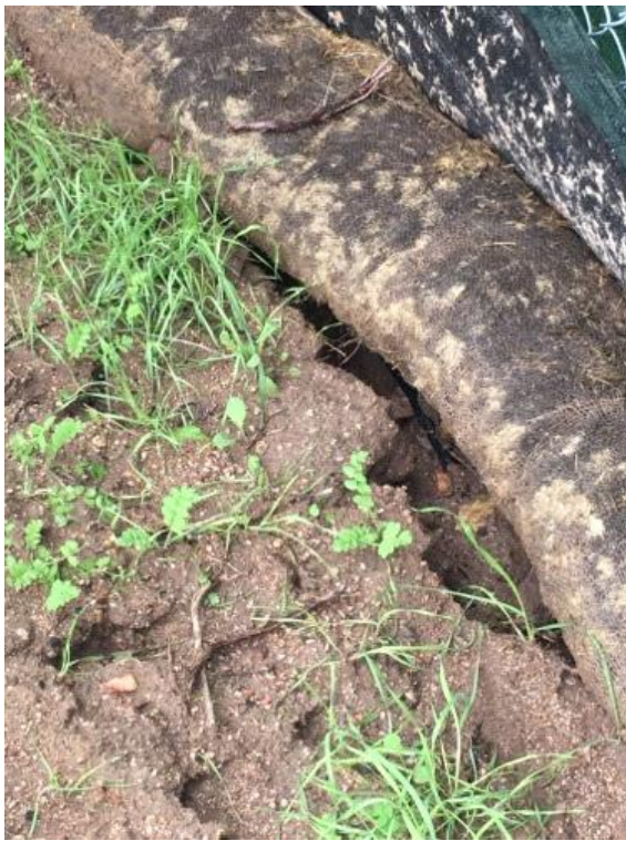
Caption Silt fence repair needed
