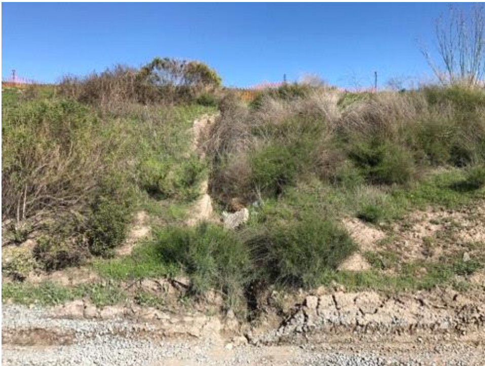
Caption Area between two transmission access roads where MPR #7 rock will be installed.
