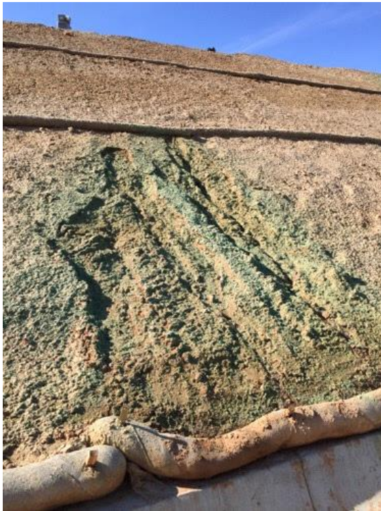
Caption Erosion rills on NE slope by construction trailer.
