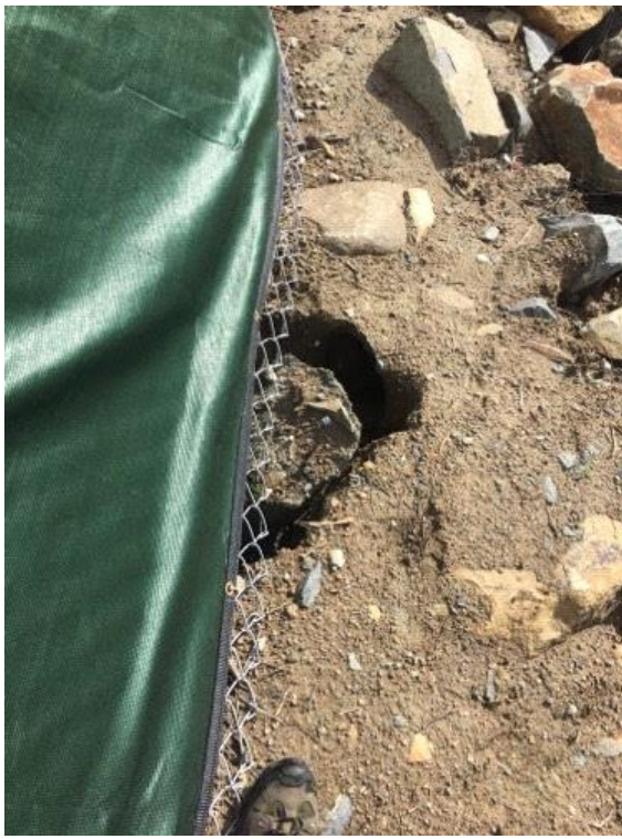
Caption Erosion at primary outfall area
