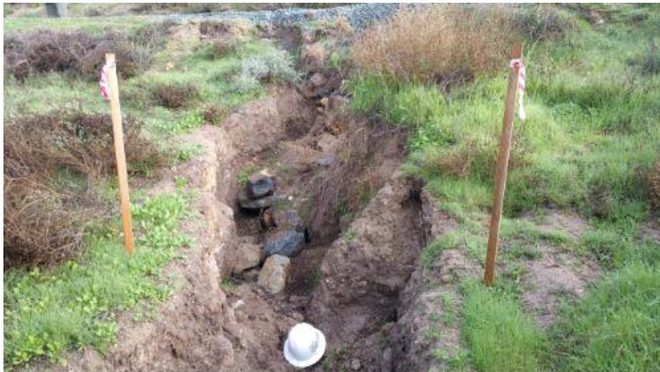
Caption Gully to east of site has not been repaired.
