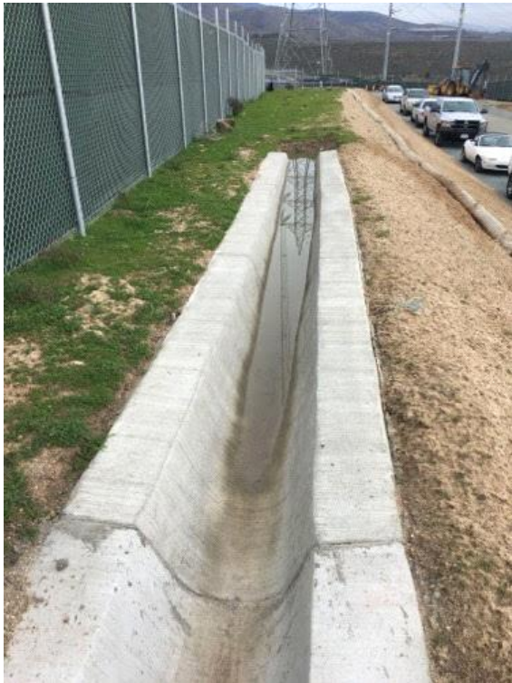
Caption Brow ditch with water along eastern boundary
