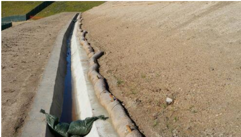
Caption Sediment buildup behind lowest row of fiber rolls on west slope was removed.
