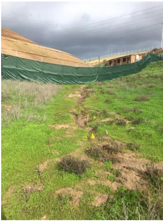
Caption Secondary outfall with flowing water within small channel Photo Attributes Capture Date/Time: Tue Jan 24 2017 10:13:34 GMT-0800 (PST) Coordinates: 32.618498, -116.948191 View Direction: Northeast
