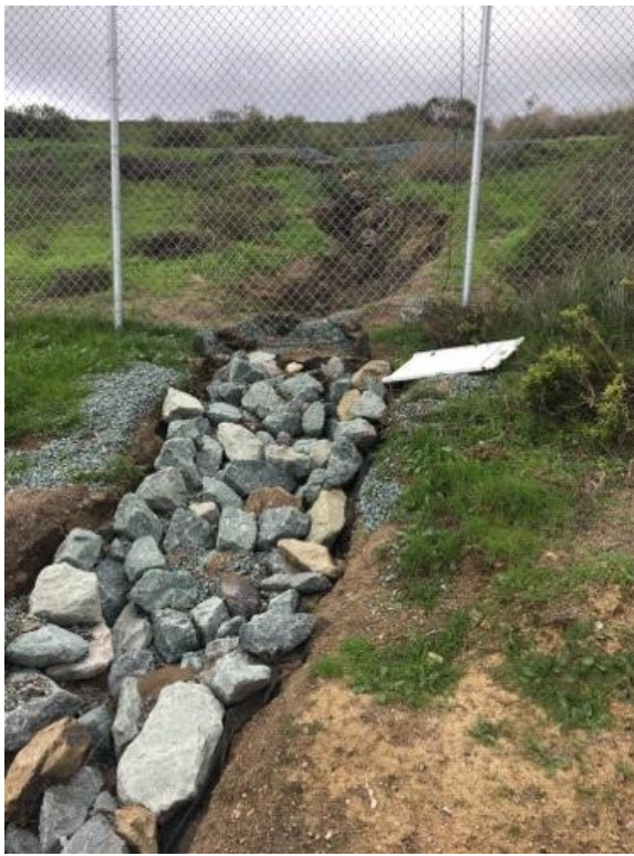
Caption Access road erosion area
