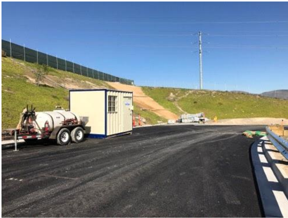
Caption First layer of asphalt on Access Road A. New security trailer.
