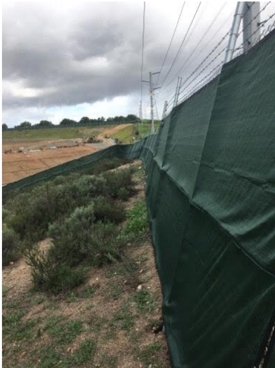
Caption Fence post failure
