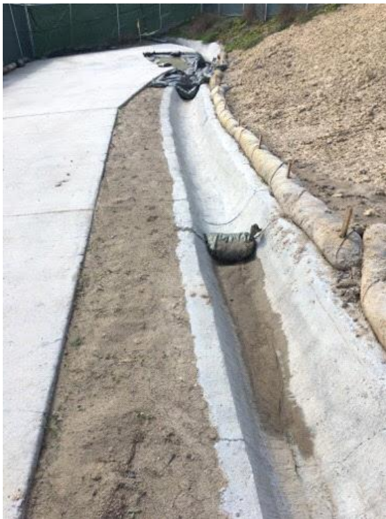
Caption Sediment near outfall should be removed before next storm.
