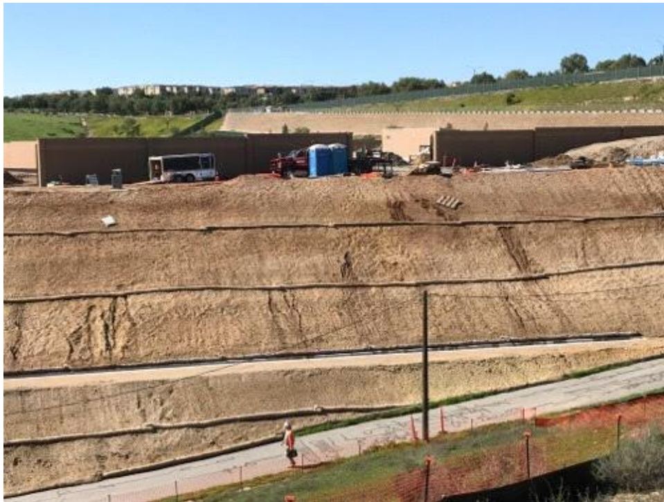
Caption Erosion on east slope.
