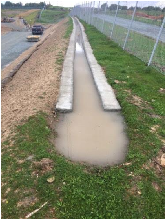
Caption Brow ditch with no outlet
