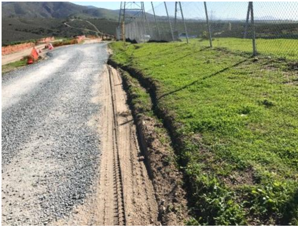
Caption Area where first truck drove off transmission access road.
