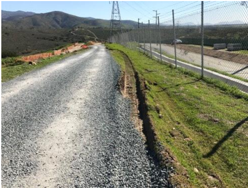
Caption Area where second truck drove off lower transmission access road.
