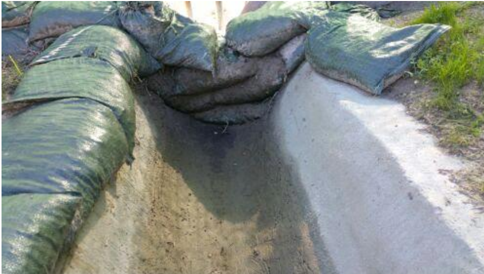
Caption Silt to top of gravel bags at bottom of main brow ditch, indicating that they may have been overtopped.
