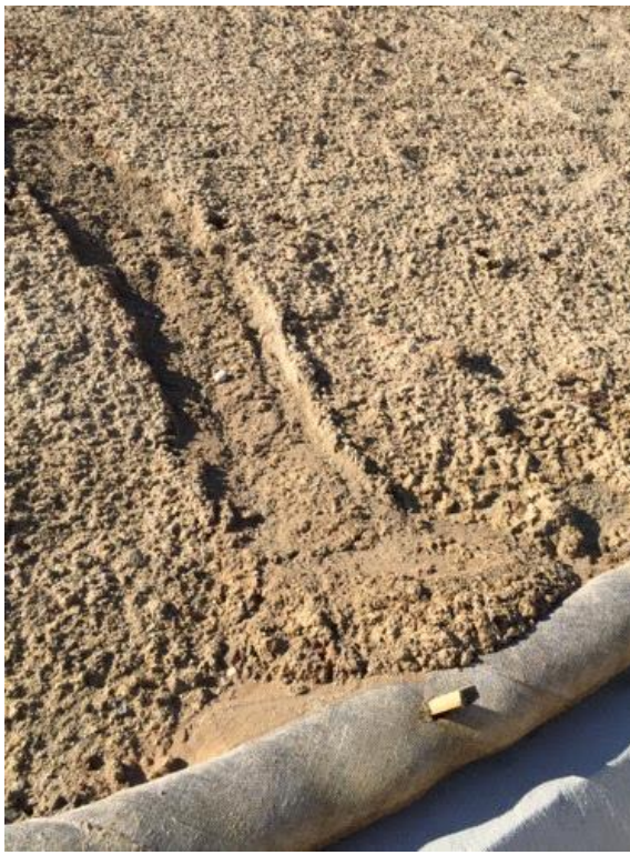
Caption Straw wattle compromised by soil buildup on NE slope by construction trailer.
