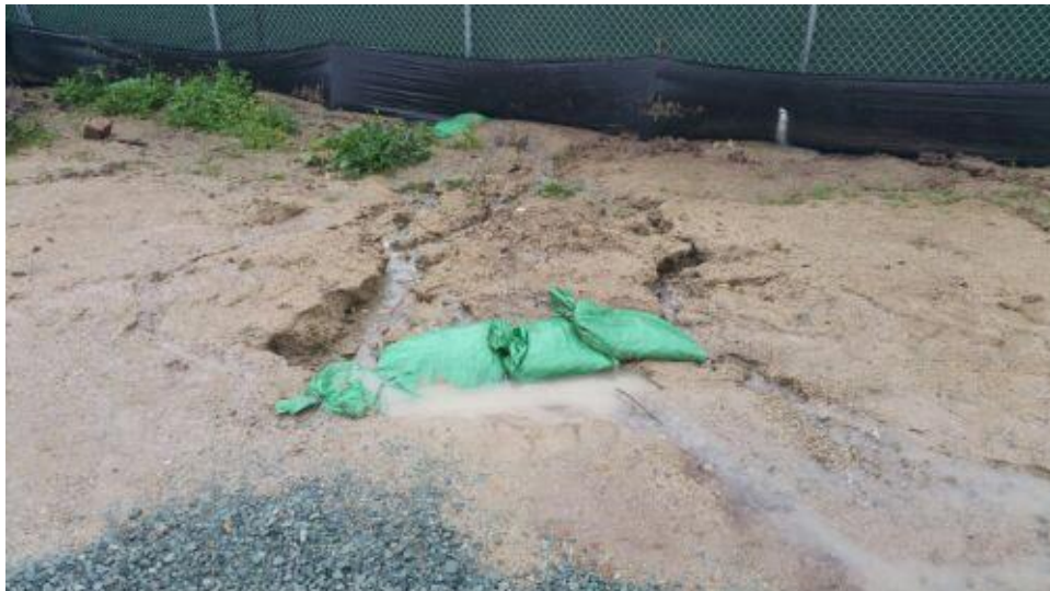
Caption BMPs for runoff from side of east entrance road have been circumvented.
