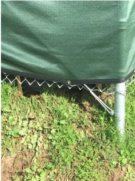
Caption Water flow evidence - matted down grass and minor erosion Photo Attributes Capture Date/Time: Tue Jan 24 2017 10:10:55 GMT-0800 (PST) Coordinates: 32.618144, -116.948652 View Direction: Northeast
