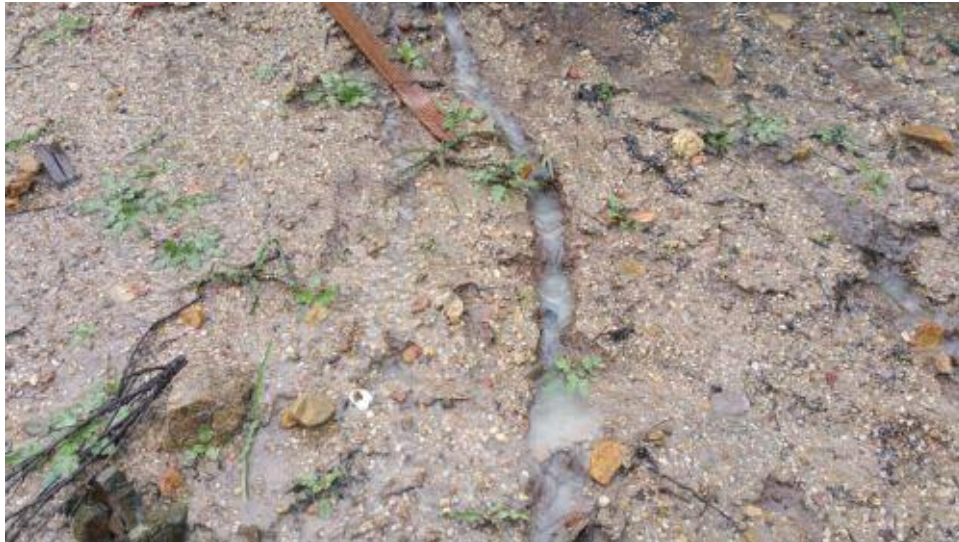
Caption Sediment-laden water running off-site down from spot where gravel bags were circumvented.
