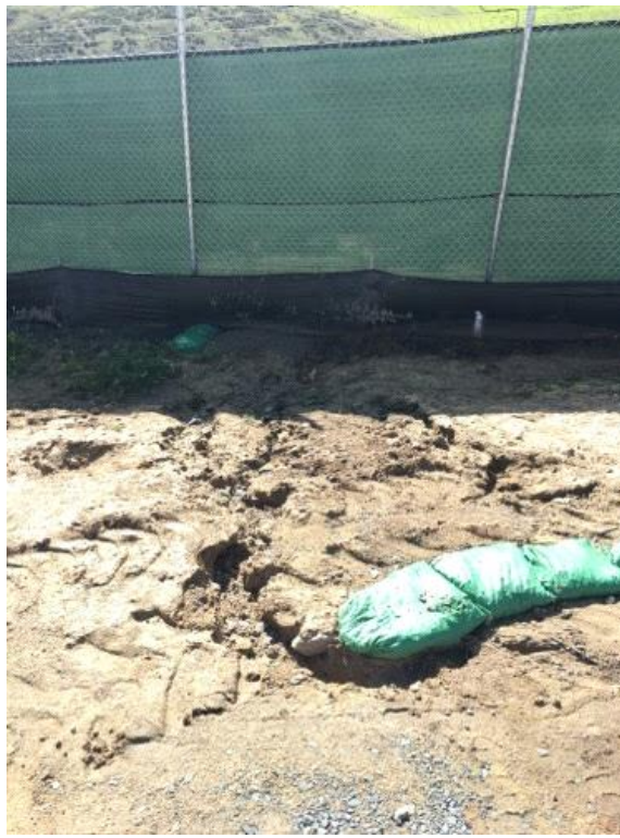
Caption Erosion near entrance, maintenance required
