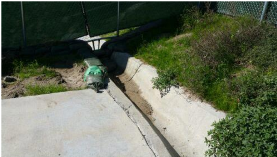
Caption Relatively little sediment build-up behind gravel bags at outflow on west end of site.
