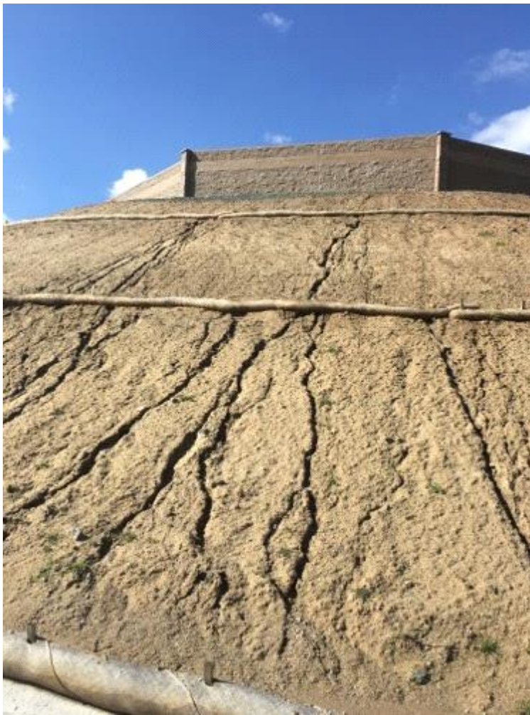
Caption Minor erosion rilling Photo Attributes Capture Date/Time: Tue Feb 28 2017 14:56:42 GMT-0800 (PST) Coordinates: 32.620735, -116.961538 View Direction: North
