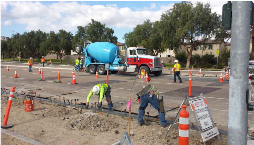
Photograph 2: Hunte Parkway curb and gutter concrete pouring occurred during the week of February 25, 2017.
