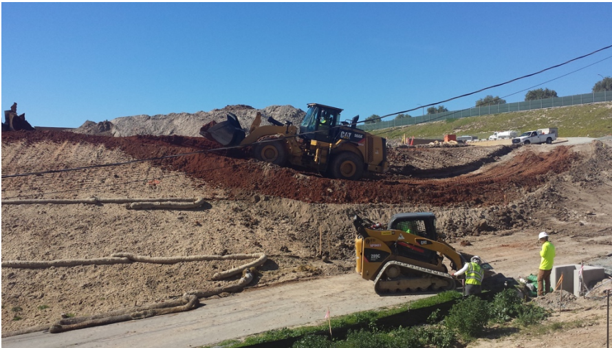
Photograph 2: Grading the ramp area between the substation and the transmission access road occurred during the week of February 4, 2017.
