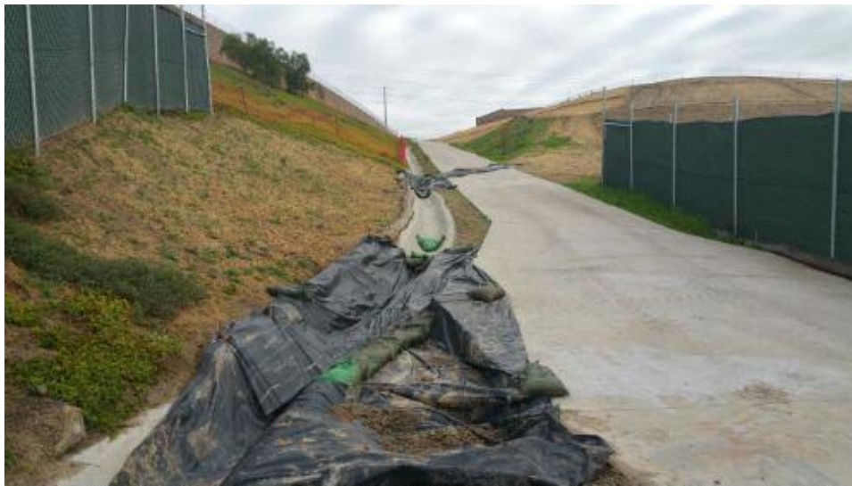
Caption Main brow ditch has minimal sediments.
