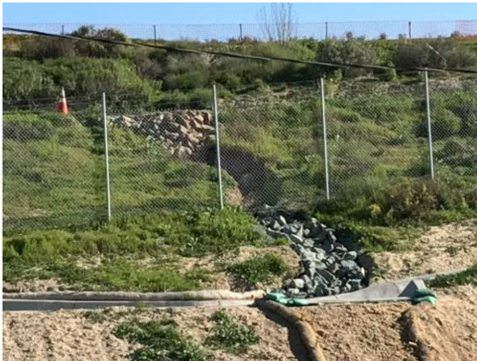
Caption Riprap placed in gully along lower transmission access road to prevent erosion during next storm.
