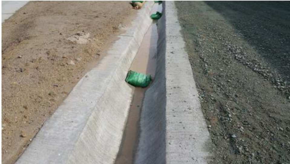
Caption Sediment-laden water flowing past gravel bags in brow ditch draining into detention basin (north side of yard).
