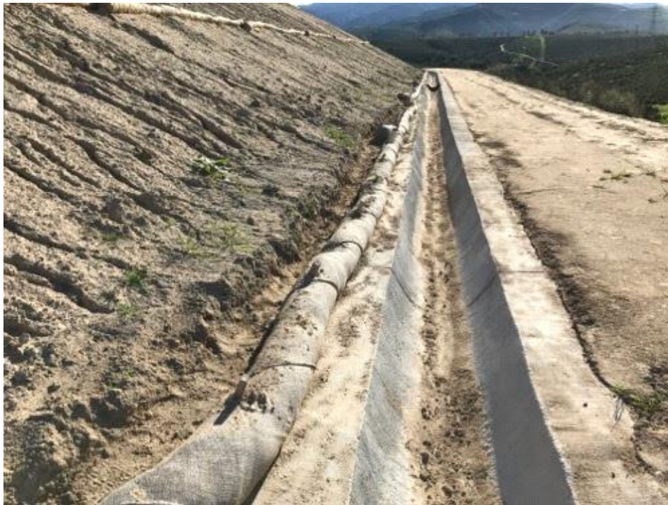
Caption Fiber rolls maintained and brow ditches cleaned in preparation for upcoming storm.
