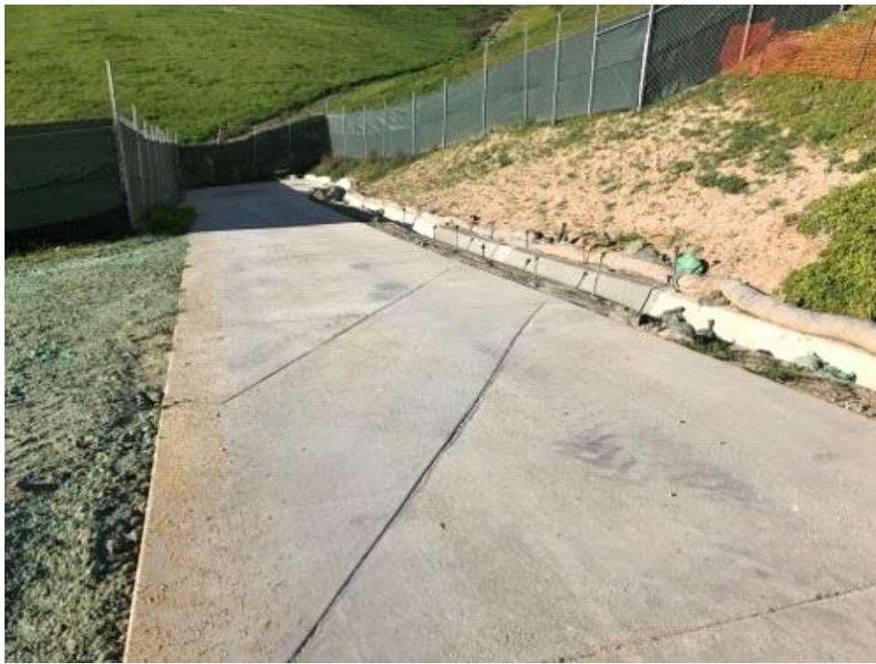
Caption Section of road and brow ditch on north side have been repaired.
