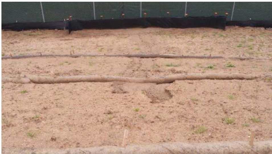
Caption Erosion has undercut two sets of fiber rolls on south slope; note double fencing installed below it.
