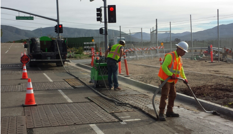
Photograph 1: Saw-cutting the pavement on Hunte Parkway for curb and gutter installation occurred the week of February 25, 2017.
