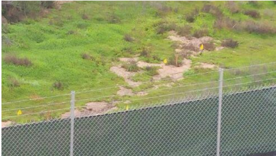
Caption Sediment deposit outside of southern side outflow has expanded from previously marked limits.
