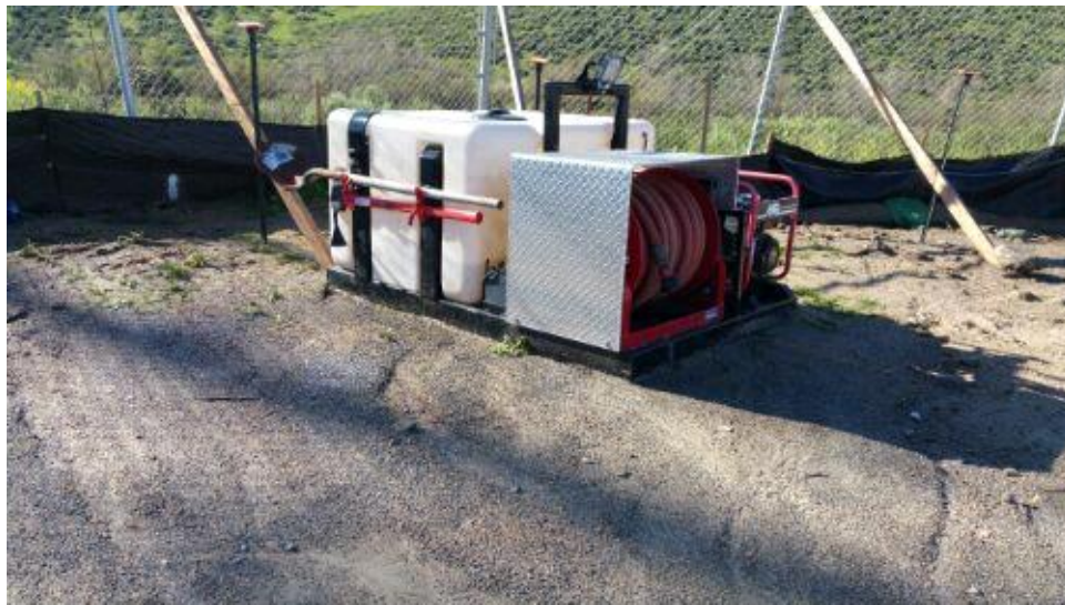
Caption Fire-fighting set-up near east entrance.
