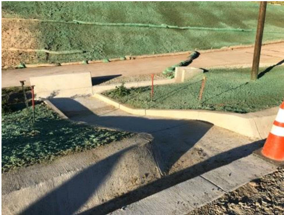
Caption New brow ditch spillway on east side of project adjacent to access road.
