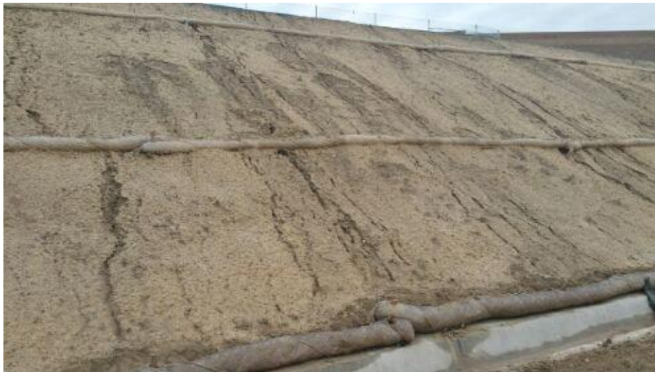
Caption West-facing slope: sediment has been removed from brow ditches and from above fiber roll.
