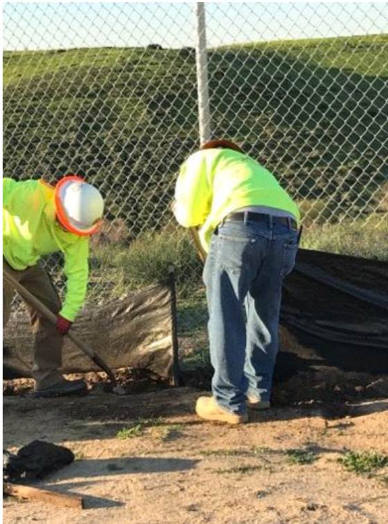
Caption Silt fence repair along upper east side access road.
