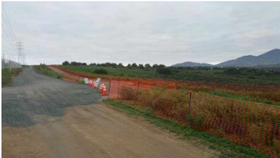
Caption Orange fencing has been repaired.
