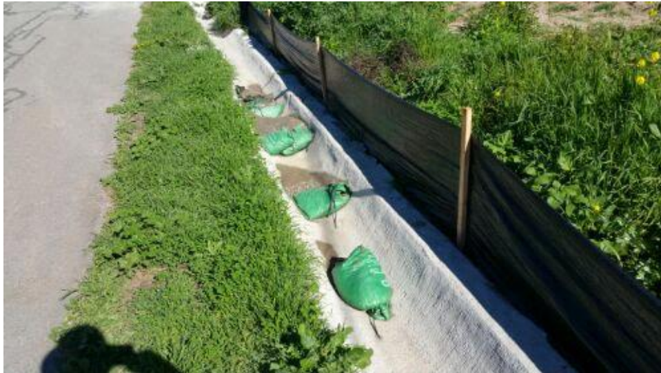
Caption Significant sediment capture in upper portion of brow ditch that goes behind trailer.
